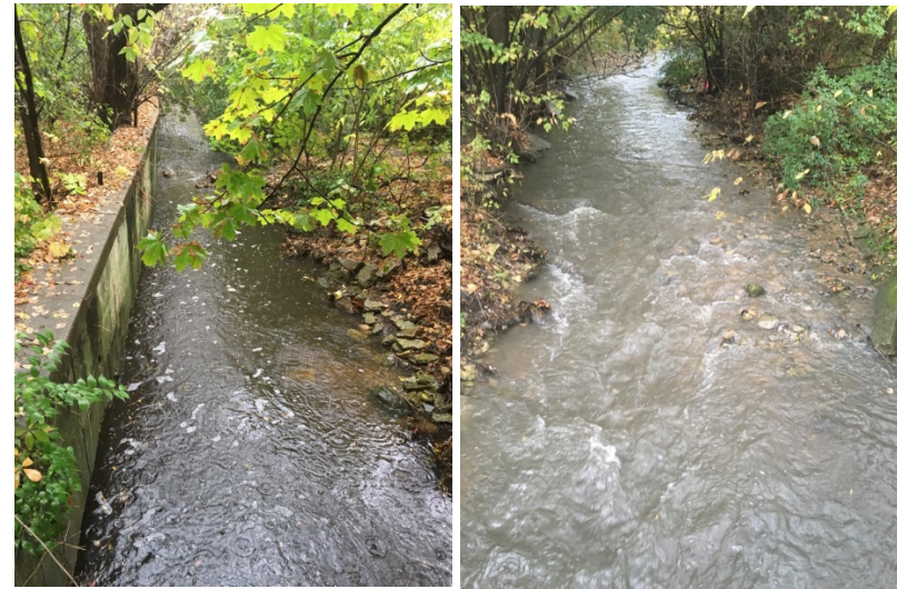
State Street Creek (left) and 7 th Avenue Creek (right) conditions during sampling on October 26 th , 2016
