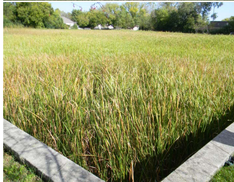
Top: typical wet bottom basin at Foundry Business Park Sportsplex; Bottom: typical wetland bottom detention at Foundry Business Park
