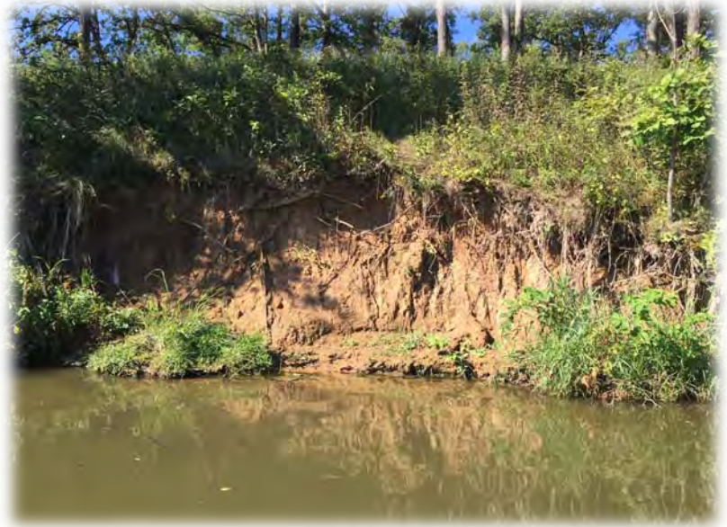
Waverly Lake; Severe Shoreline Erosion
