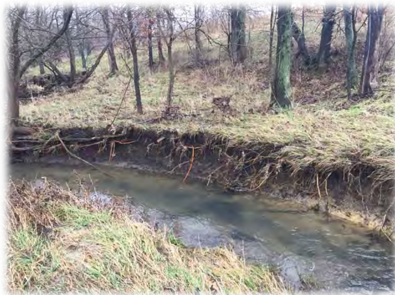
Woods Creek; High Bank Erosion
