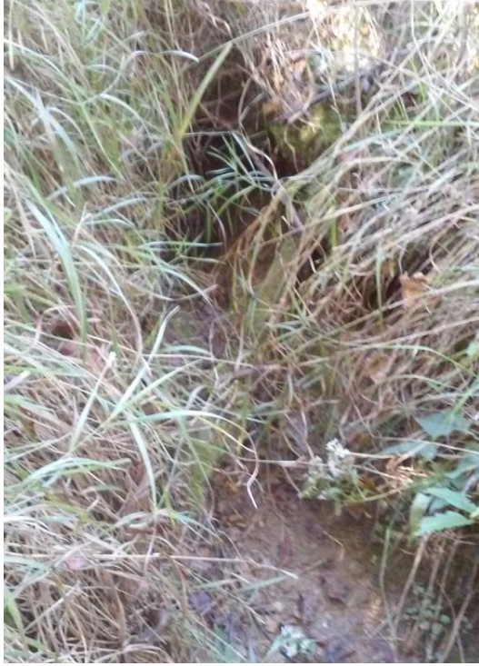
Figure 13. Site 3 middle channel erosion.
