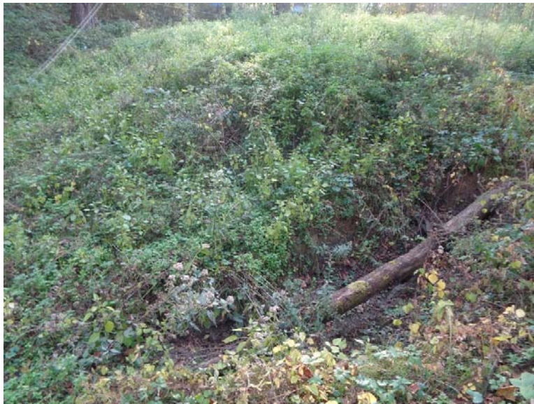
Figure 30 Downstream side of channel being washed away at Structure 21.
