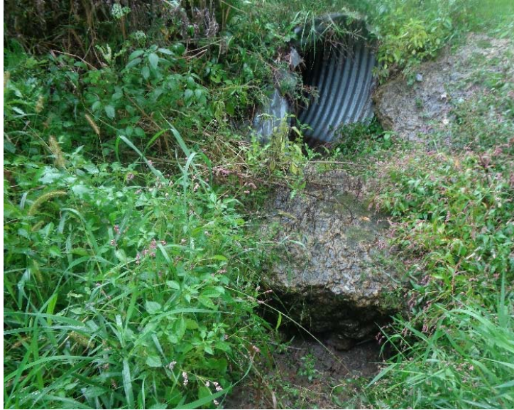
Figure 11 Erosion occurring downstream of Structure 11.
