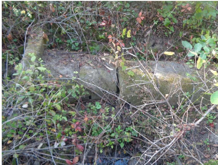
Figure 31 Structure 22 failed reinforced concrete pipe.
