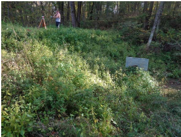
Figure 28 Upstream side of Structure 21 with trash rack overgrown with vegetation.
