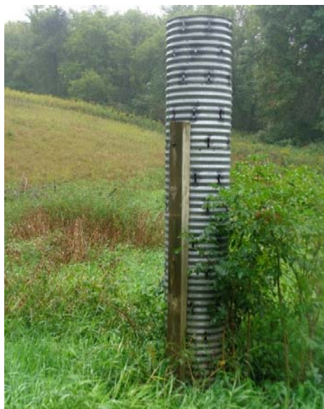
Figure 4 Corrugated riser with 1 inch by 3 inch slots.
