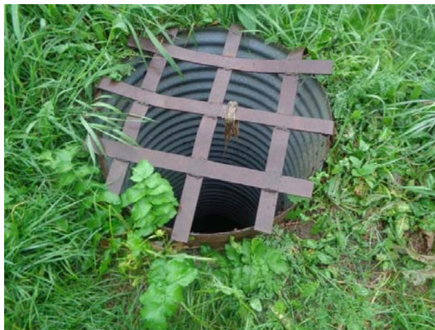
Figure 14 Grates on Structure 12 dry dam to block large debris.
