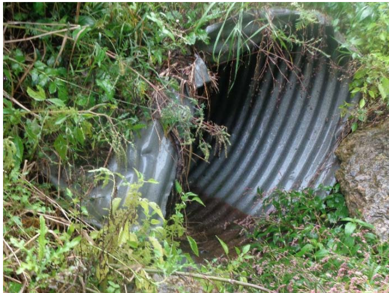
Figure 10 Culvert damage downstream of Structure 11.
