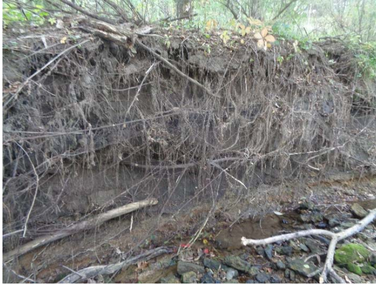
Figure 6. Upstream erosion at Structure 7.
