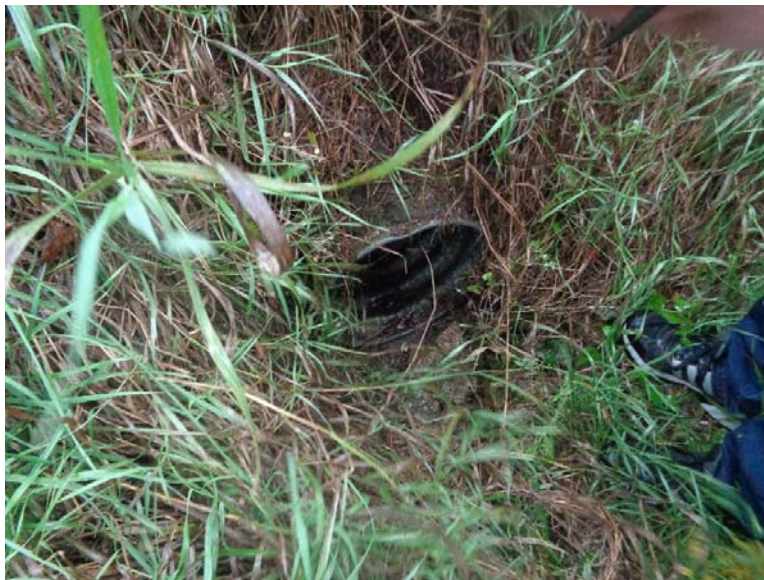
Figure 8 Structure 8 upstream corrugated pipe with overgrown vegetation pulled back.
