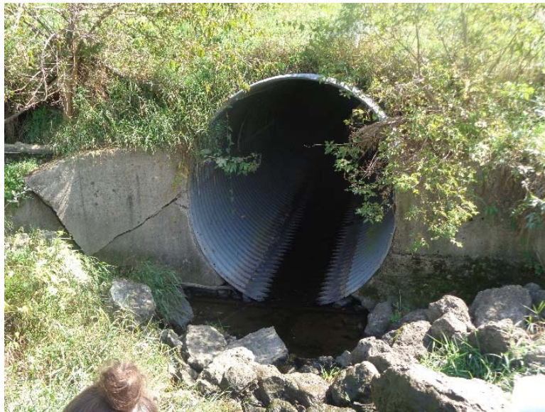
Figure 21 Cracked abutment Structure 18.
