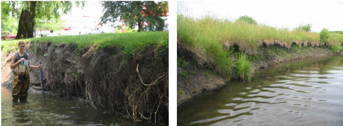
Figure 20. Examples of a high degree of bank erosion along Boone Creek in reach 3 (left) and reach 9 (right) observed during a 2002 stream assessment.
