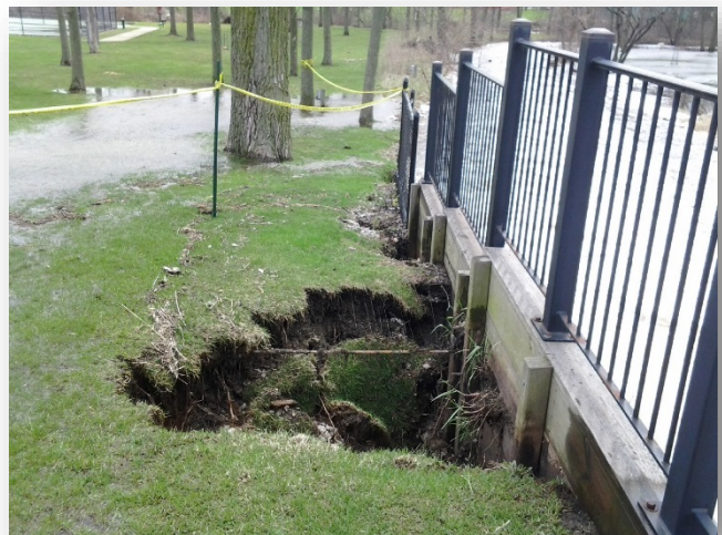
Figure 5-5: April 2013 flood event in Grandwood Park Flooding damage to the Grandwood Park Dam
