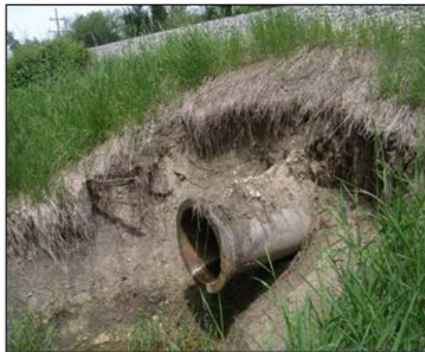
Figure 3-63: Example of a discharge point
