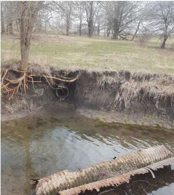
Photo 17: Tile outlet on eroding bank in a pasture on North Branch above Duroc Road. Note tile is near flowline of channel. (Reach 005)
