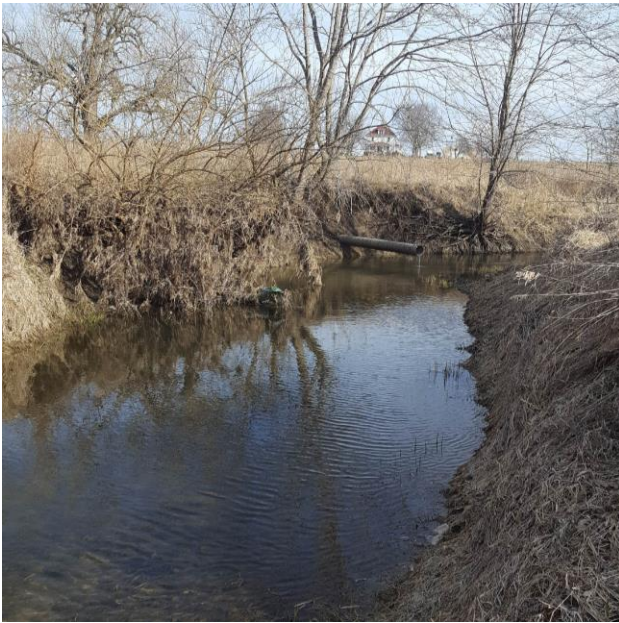
Photo 14: Upper end of Friends Creek Ditch near Rd. 000E Note length of tile outlet protruding into stream. (Reach 004)
