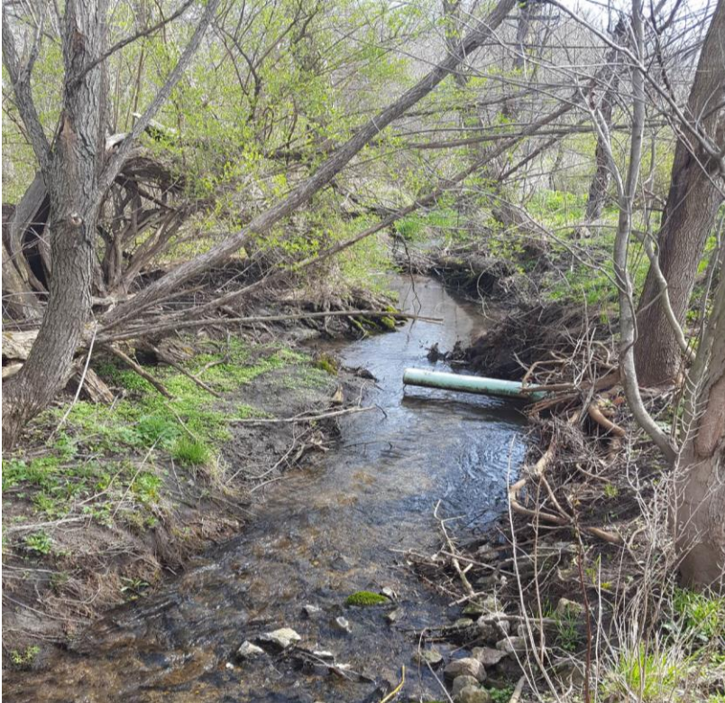
Photo 24: Upper end of Trib. 3 approx. 150 ft. upstream of headcut.
