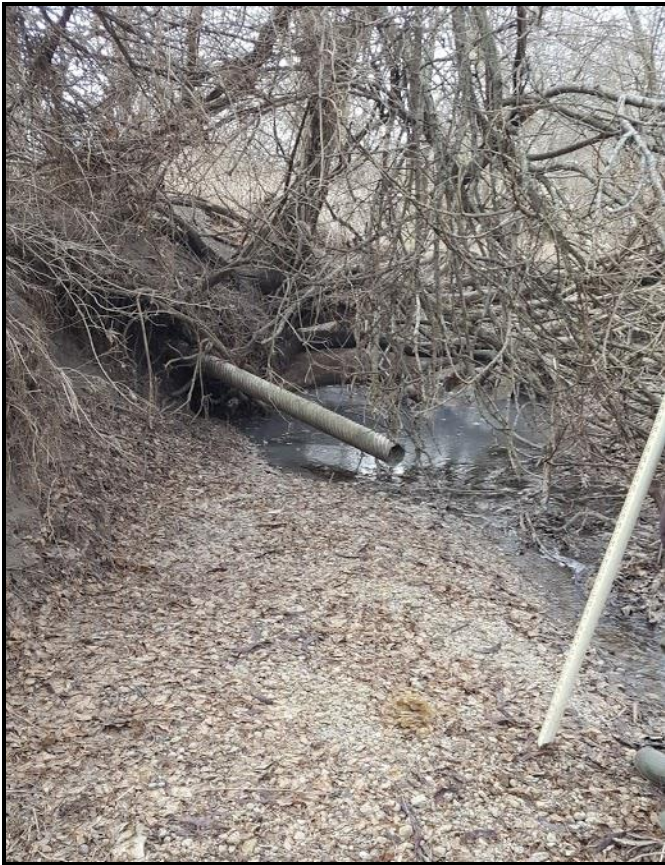
Severely Eroding bend with exposed tile outlet and fallen trees. (Reach 001)
