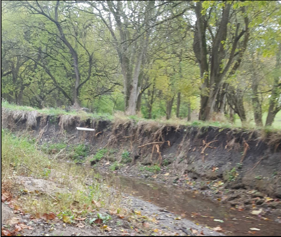
Exhibit 4---Severe Erosion: Tile outlet extending into channel, vertical bare banks and exposed tree roots.
