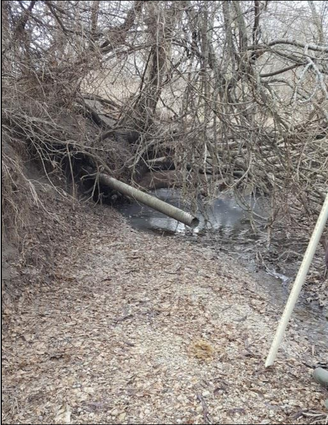
Exhibit 6---Very Severe: Tile outlet exposed 10 ft. and trees falling into channel
