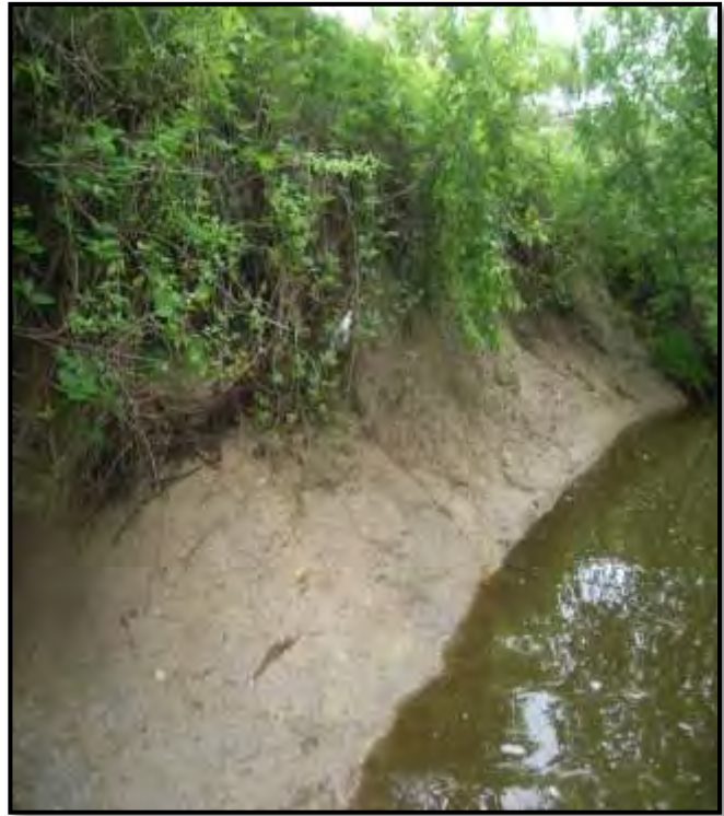
Streambank Erosion in the Avon-Freemont Drainage Ditch
