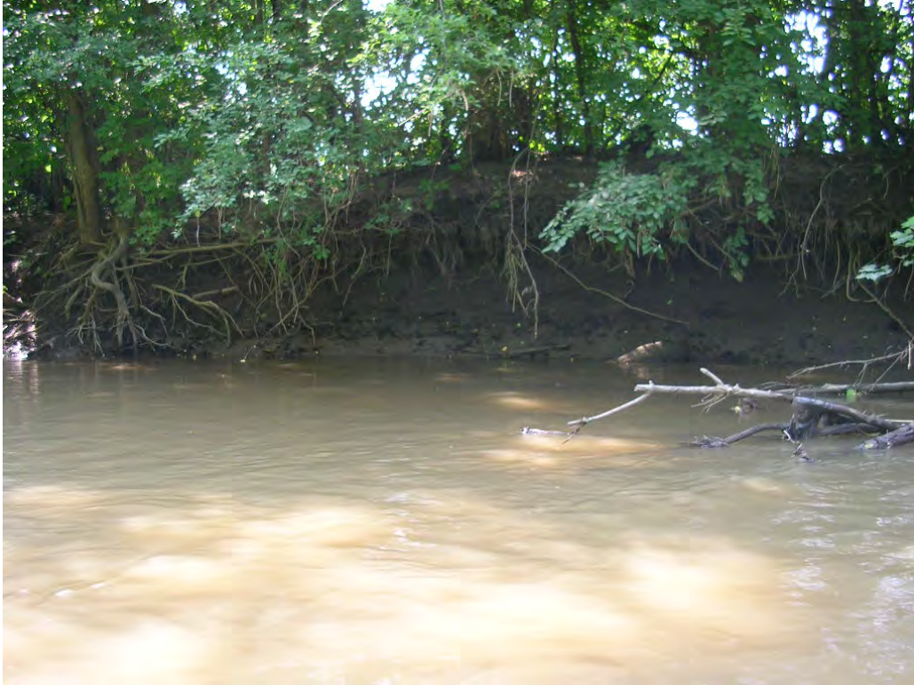
Photograph 5: View of bank erosion near Dilley's Road
