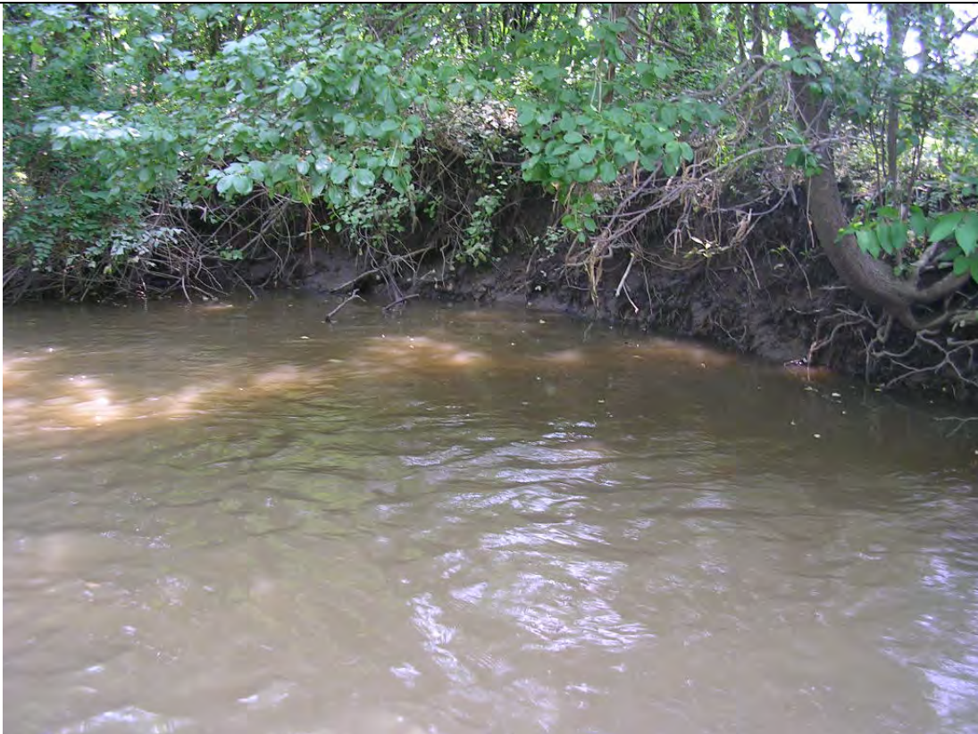
Photograph 2: Area of streambank erosion near Sampling Site/Reach 1
