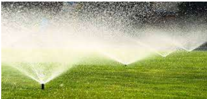
Photo 121: Example wastewater reuse spray irrigation system for turf grass.
