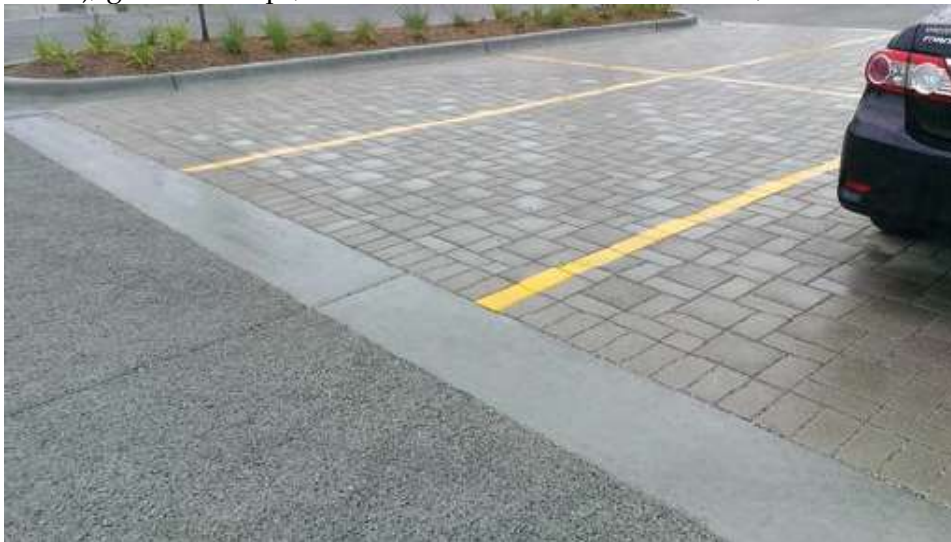
Photo 104: Example permeable pavers (right) and porous concrete (left) in a parking lot to infiltrate large volumes of stormwater runoff prior to discharge (Photo Courtesy Village of Franklin Park at the Police Station).
