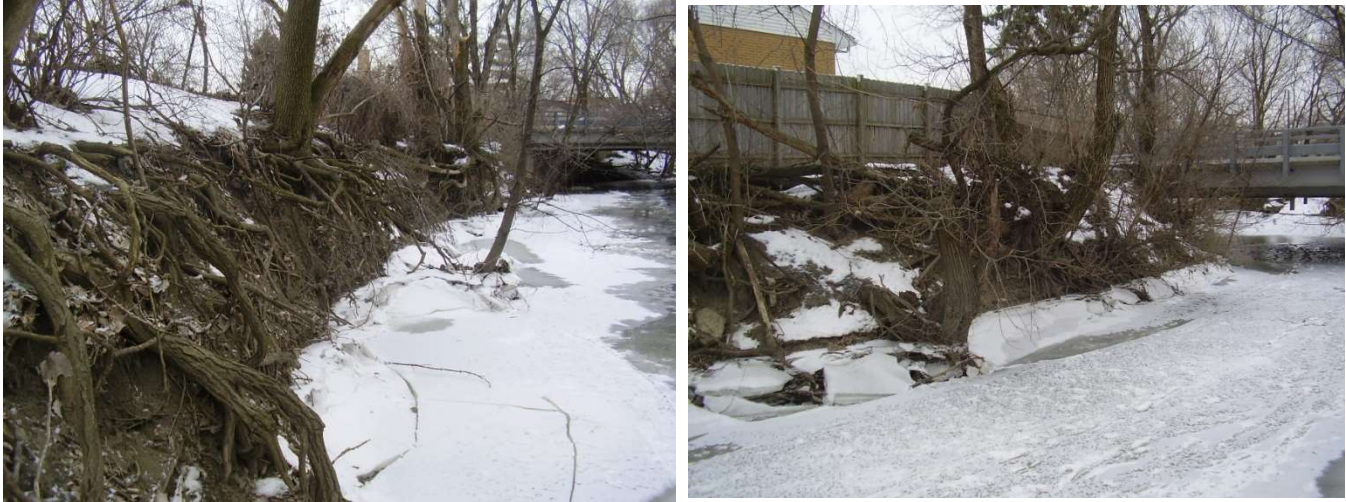
Photos 58 and 59: Streambank erosion is severe downstream of the 9 th Avenue Bridge.
