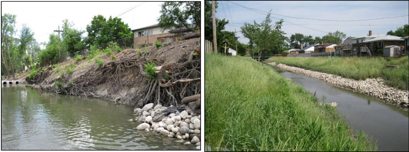
Photos 60 and 61: Before and After Photos of the Phase 3 Silver Creek Stabilization Project completed in 2010 by the Village of Melrose Park near Elsie Drive. Rock toe, re-shaped slopes, rock vortex weirs, rock riffles, and native plantings were installed. Bank stabilization can reduce loadings of pollutants such as total suspended solids, total phosphorus, and/or total nitrogen.
