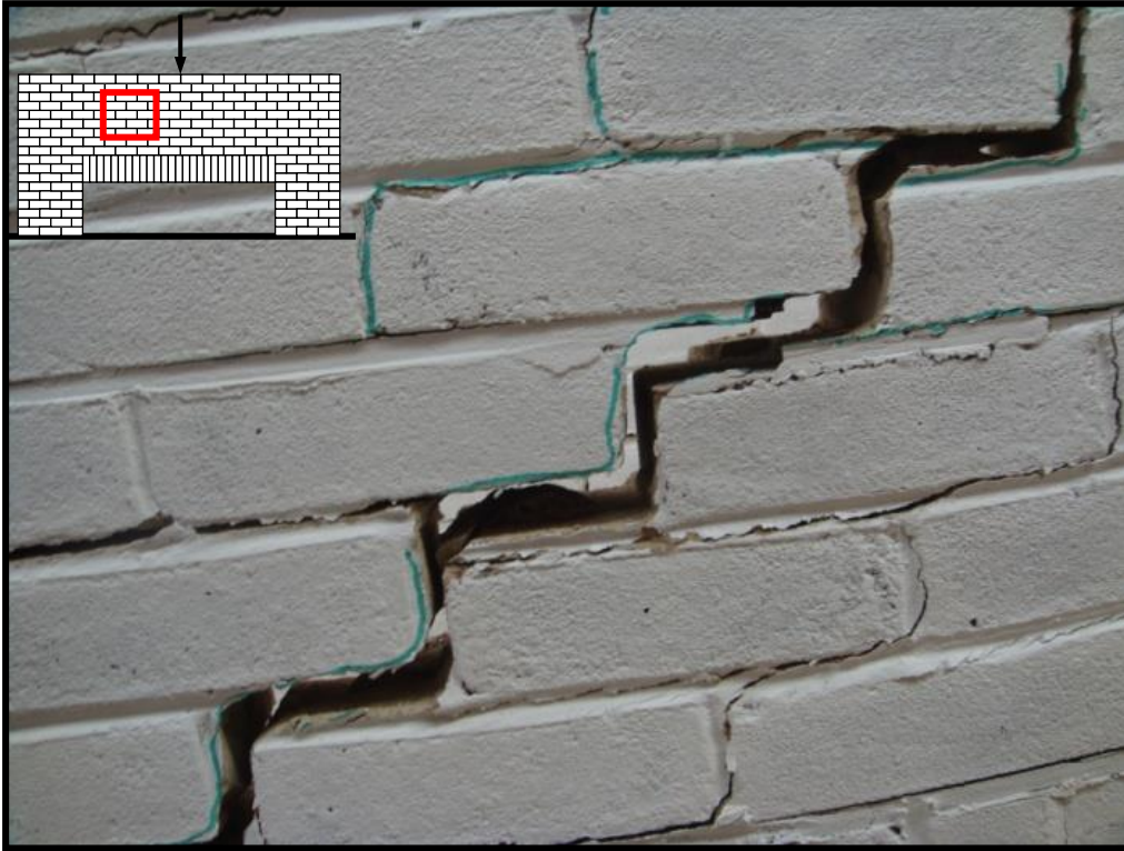
Fig. 12. Shear development propagated from the corners of the opening to the top of the panel.
