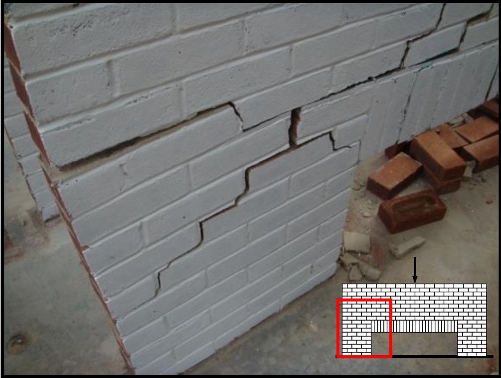
Fig. 13. Flexural crack at the right hand support.
