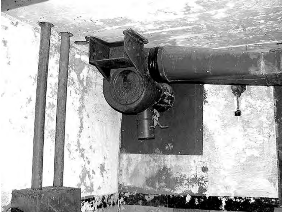
Interior of subterranean computer room at Battery Opauala's BCS showing CWS centrifugal blower motor and associated duct. Author, 2002
