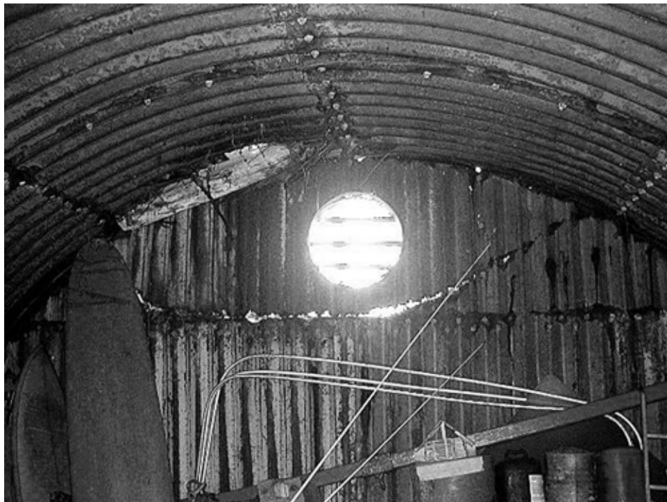
Interior of radar operating room at Battery Opaepala (Riggs), showing “elephant iron” construction. Author, 2002
