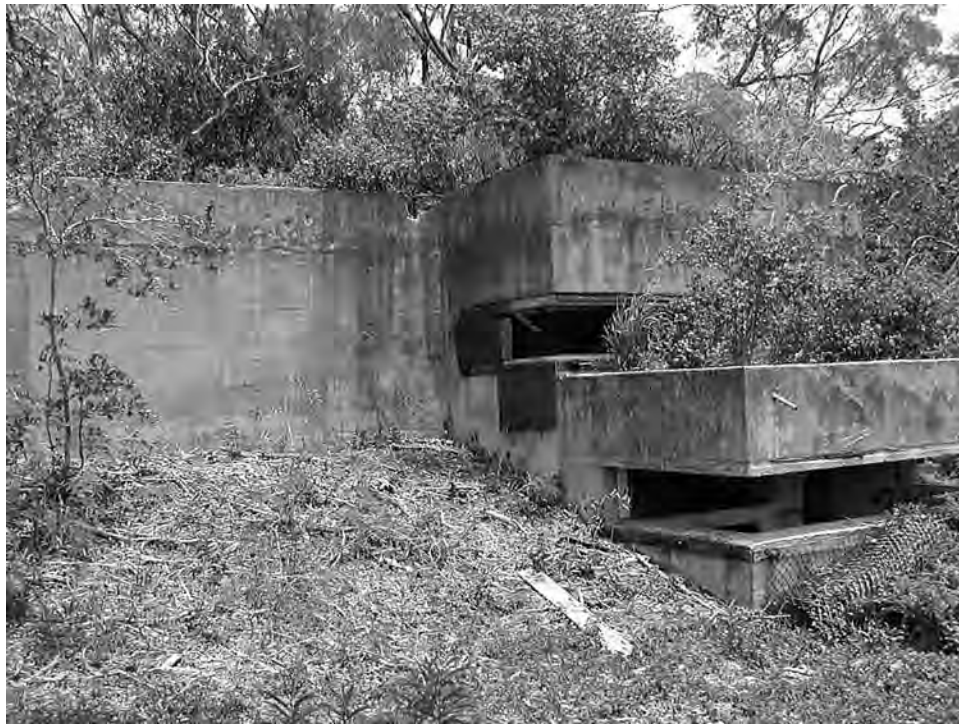
Double-tiered BCS of Battery Wilridge (Kirkpatrick) with radar operating/FCSWBD room on the left. Author, 2002
