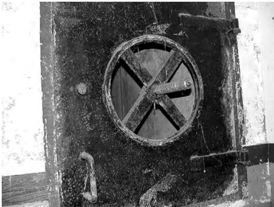
Door to escape hatch in FC switchboard room, Plotting Room No. 2, Battery Opaeula (Riggs). Author, 2002
