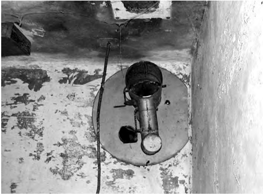
NE corner of radar operating room of Battery Wilridge (Kirkpatrick), showing valve connected to outside T-shaped ventilator of concrete pipe. Author, 2002
