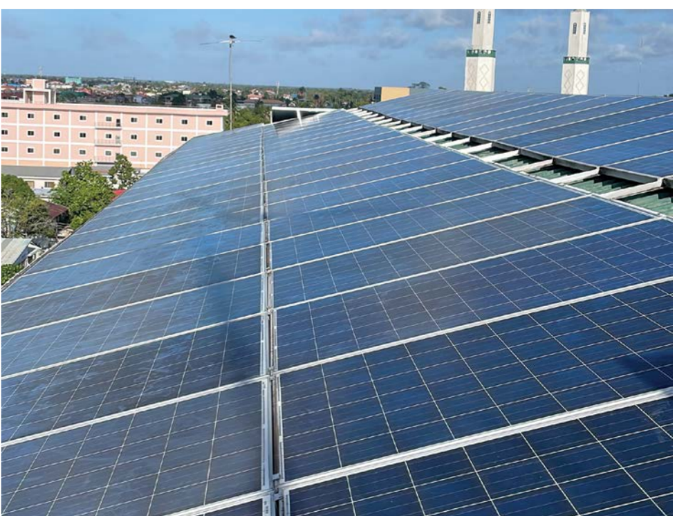
The Sleepin International Hotel generates 40% of its electricity from renewables.
