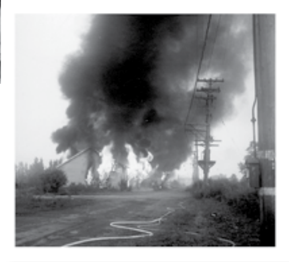
Image 189 (inset): Initially, NASA let the PBOW structures stand. As more and more acres were acquired, however, workers began to destroy a large number of the buildings. In 1961 a local company was hired to raze all unusable structures and to dismantle three acid plants. However, a number of the nonmanufacturing structures were retained (GRC-2015-C-06565).
