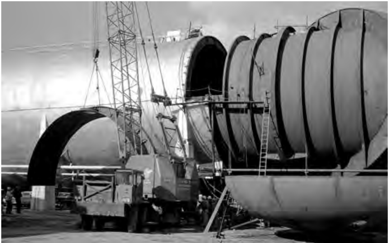
Image 191: Three bulkheads were placed inside the AWT to create the SPC. The largest is seen here being inserted approximately where the wind tunnel fan was located (NASA C-1961-58551).
