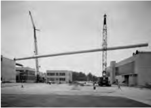
Image 144: The overhead air-handling line between the PSL and the 8×6 is installed in 1954 (GRC-2007-C-025662).
