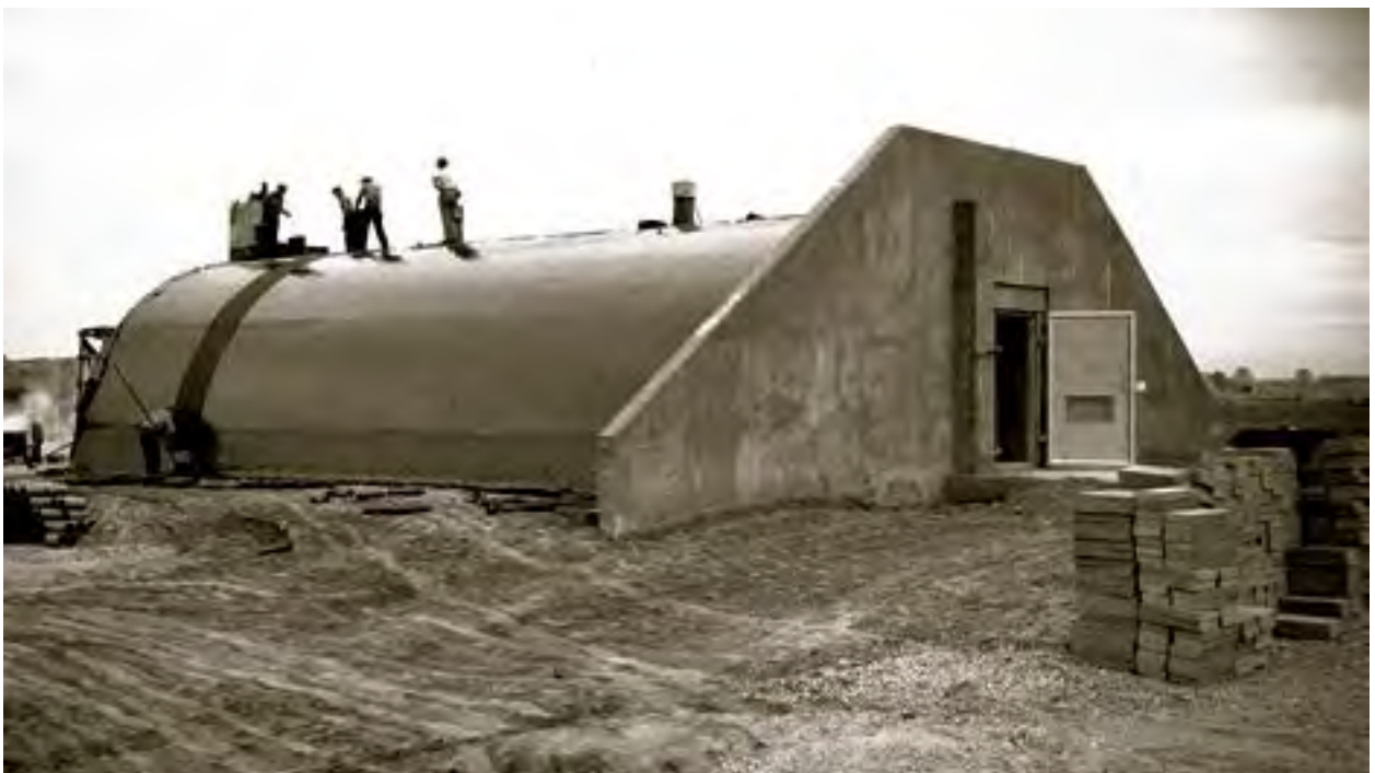
Image 29: Construction of one of the 99 concrete bunkers used to store explosives, c1941 (GRC-2015-C-06817).
