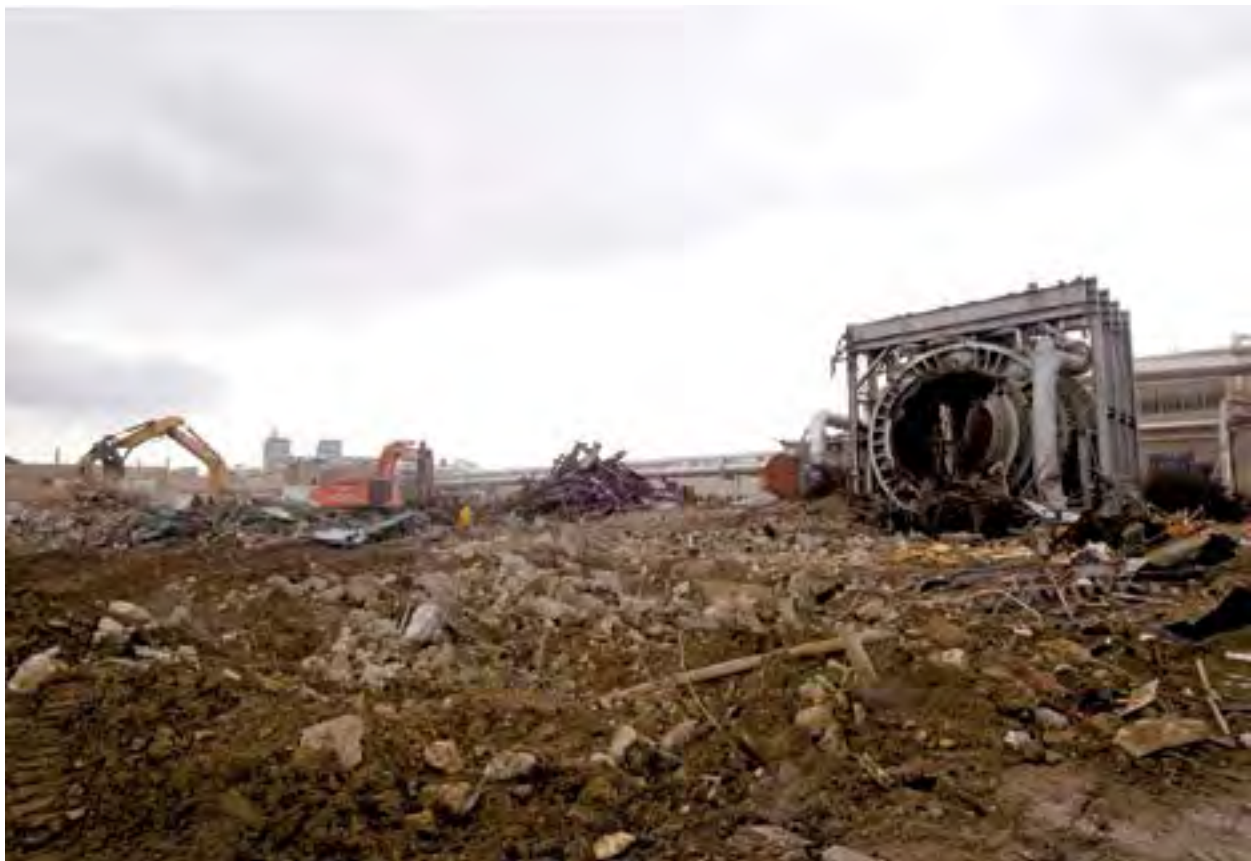
Image 394: PSL wasteland in July 2009. In just over two months, the wrecking crew leveled a facility that had been part of the center's landscape for nearly 60 years (GRC-2009-C-02018).
