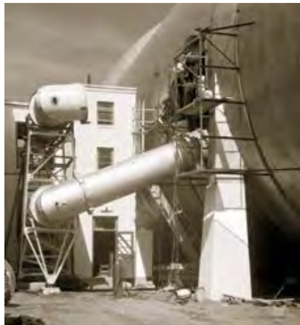
Image 112: Construction of the lab's first supersonic tunnel. Eventually the building would house three small supersonic tunnels (GRC-1945-C-10764).
