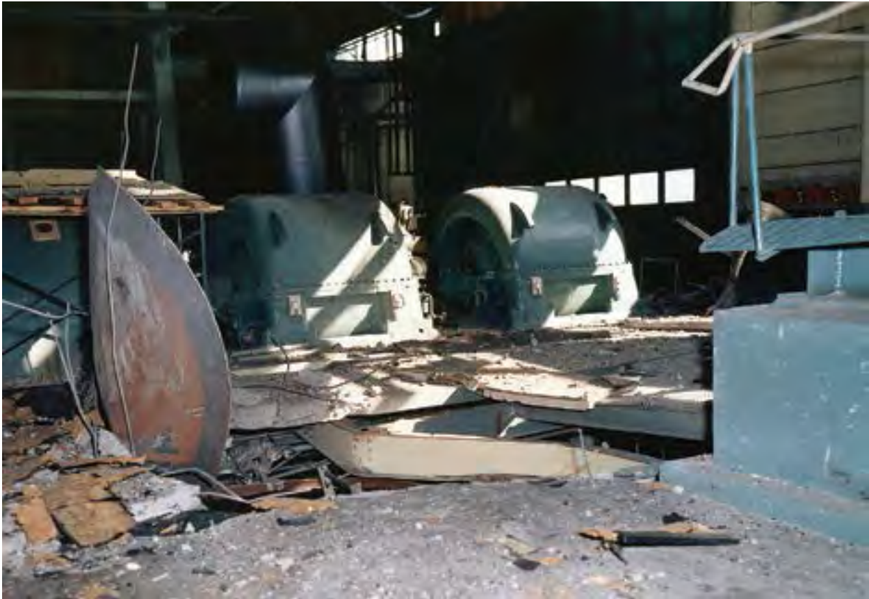
Image 241: Damage to the PSL Equipment Building (GRC-1971-C-01422).
