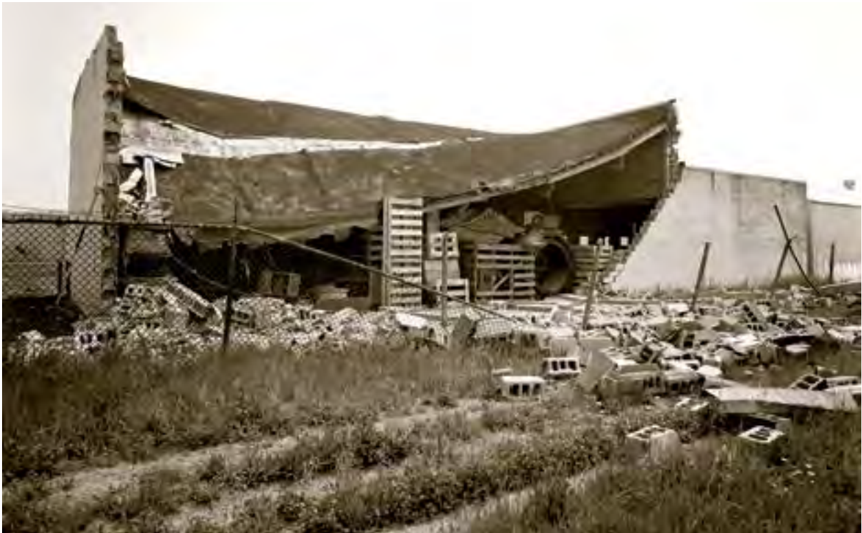
Image 136: Tornado damage included a collapsed roof on the Trunnion Building (GRC-1953-C-32966).
