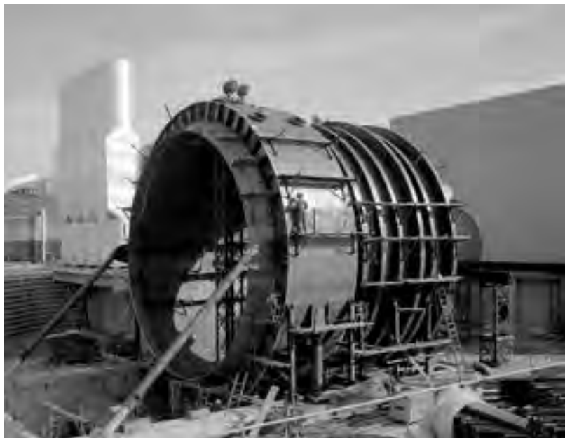
Image 216: Construction of the 50-foot-diameter cooler for PSL No. 3 and 4. The cooler contained 5,500 water-fed cooling tubes and three banks of spray nozzles to reduce the engine exhaust temperature from 3,500 to 120 degrees Fahrenheit (GRC-1969-C-03898).
