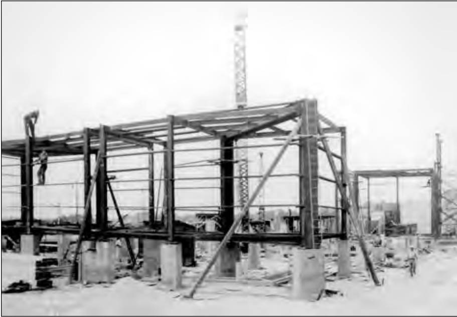
Figure 2-3. Shell framing for the Icing Research Tunnel, with Altitude Wing Tunnel in background, 21 July 1943. (NACA C-IRT-4)
