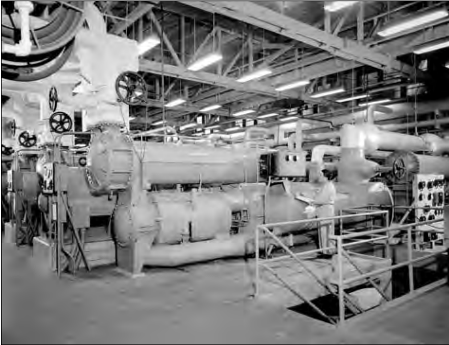
Figure 4-8. Carrier components and condensers of the refrigeration plant, 5 February 1950. (NACA C-25219)
