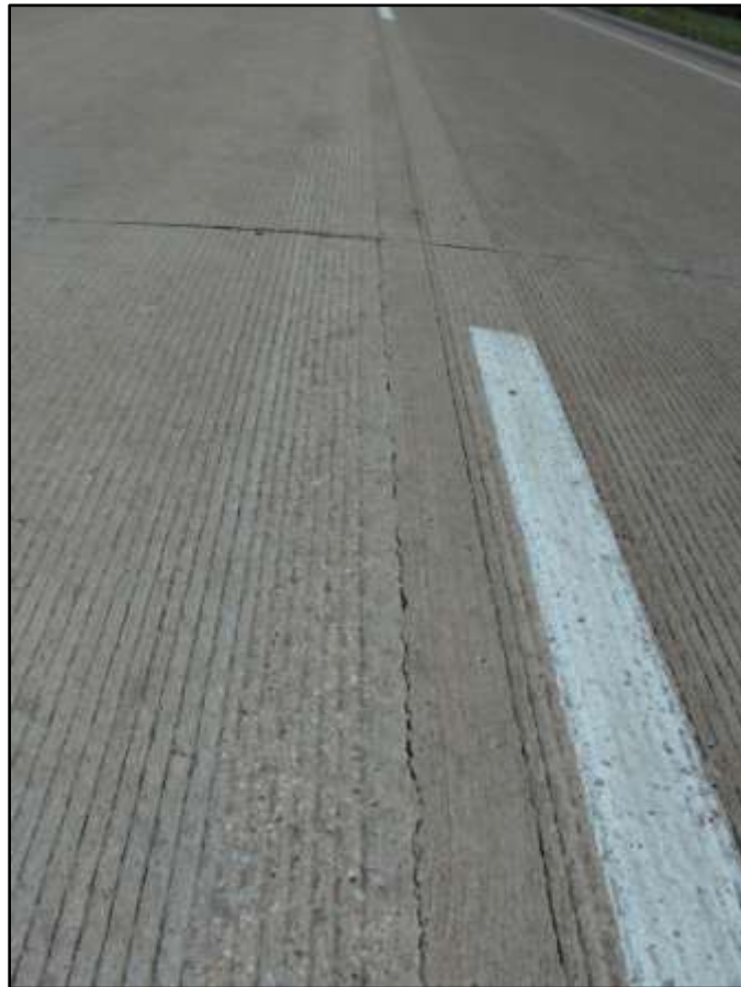
Figure 62 - Hairline crack on knifed joint
