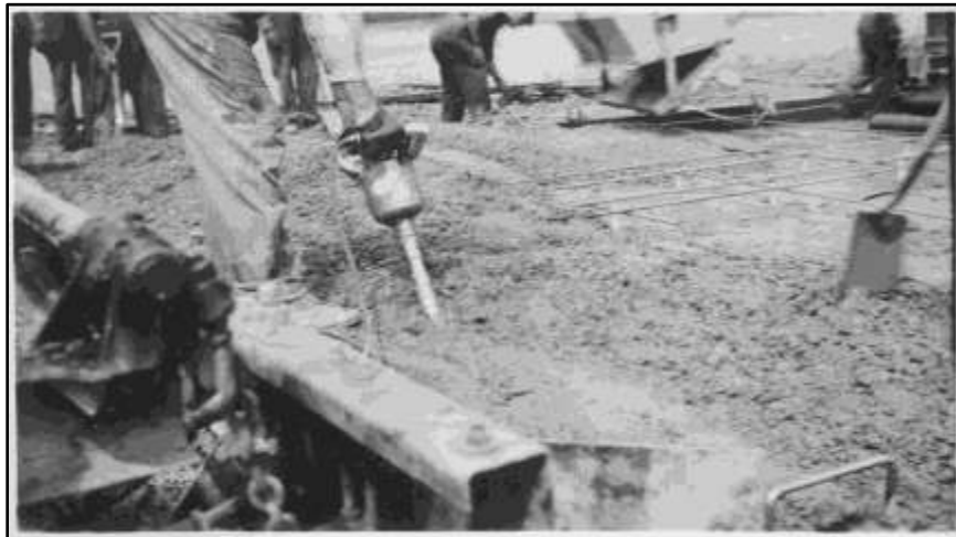
Figure 36 - Vibration near expansion joint - Bremer County 1936
