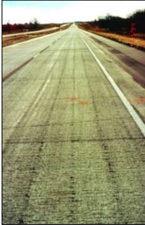
Figure 38 - Vibrator trails in pavement - Dallas County
