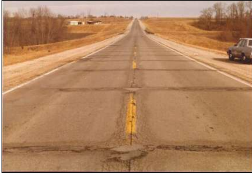
Figure 9 - D-Cracking on U.S. 218 MP 46 - 1970s
