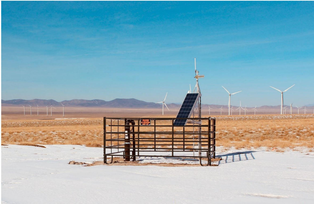
Figure 5. A previously completed seismic monitoring well.
