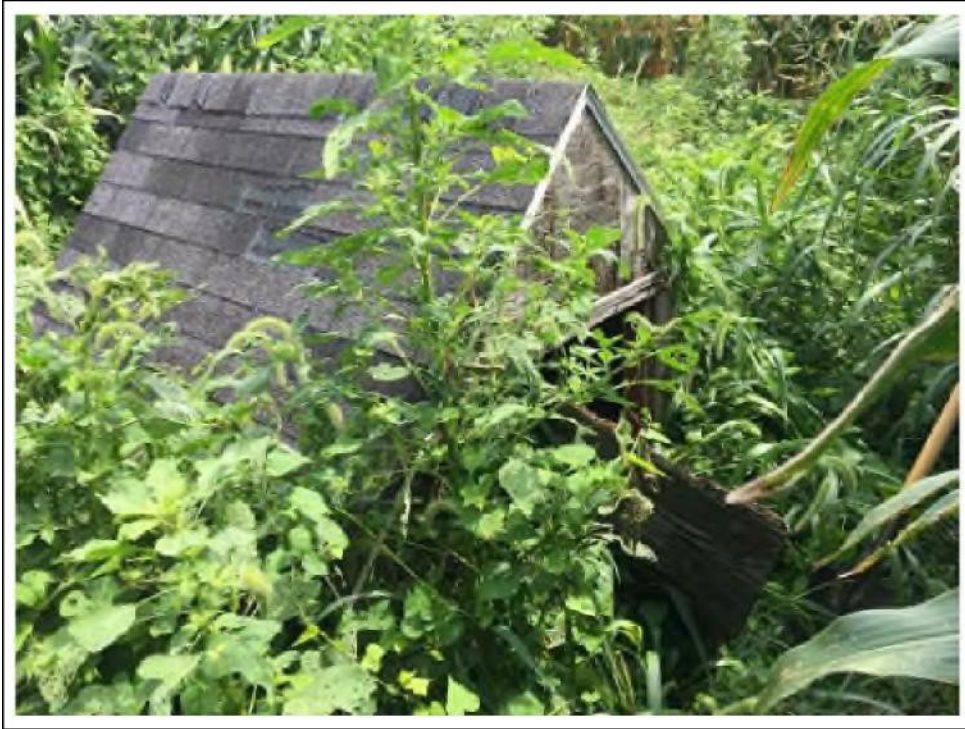
Figure 28. East Facing H-1 Pumphouse
