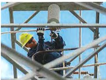
Jimmy Snider, electrician, completes work on the rebuilt Oklee substation in northwest Minnesota. Minnkota budgets to rebuild two of its aging distribution substations annually.
