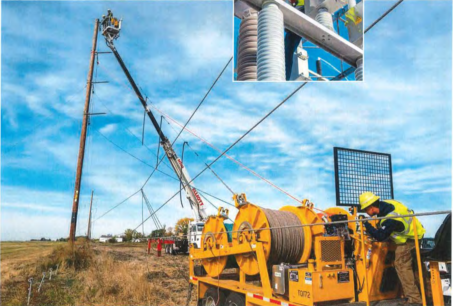
From ground level to the top of a transmission structure, Minnkota crews string wire on a rebuilt section of 69-kV line near Cavalier, N.D.
