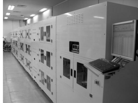
Automated inspection and formation
