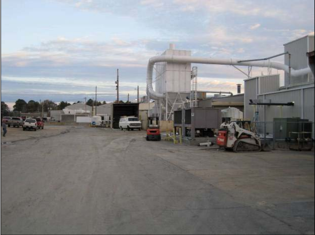
Figure 2-6. View of the south side of the proposed Columbus project area. Exide would remove the baghouse, demolish the building to the right, and then construct the addition in this area.
