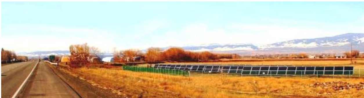
Figure 3-3. Current view of solar panels at the City of Ellensburg's Renewable Energy Park along the eastern side of I-90.
