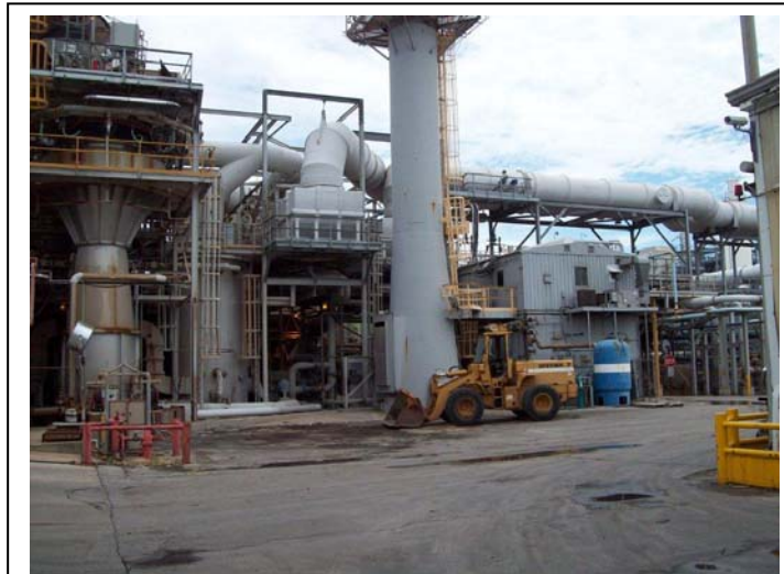
Figure 1-1. CHDP Facility Incineration Train I
