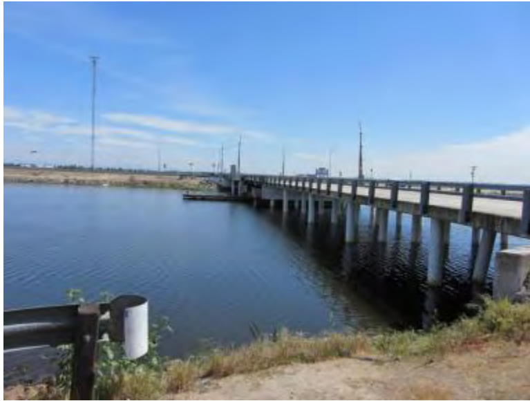
Photograph 9. Bishop Cut at Eight Mile Road Bridge. Swallow nests are present under the bridge. Photograph taken April 3, 2013.
