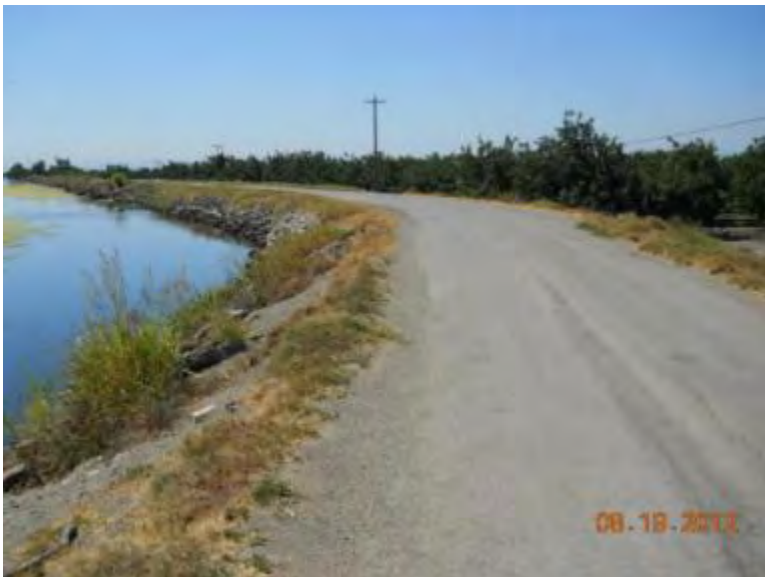
Photograph 6. King Island Road looking south. Bishop Cut is on the left. Photograph taken August 20, 2012.
