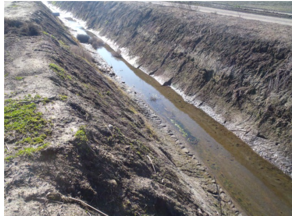
4. Denuded ditch situated approximately 450 feet west of the project site
