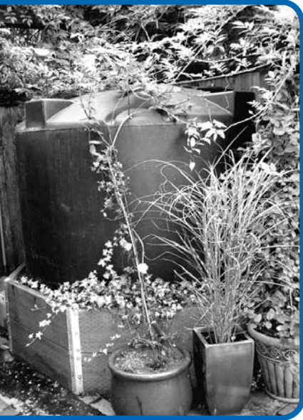
Rainwater harvesting tanks come in many shapes and sizes. This 550 gallon cistern in Eugene is elevated so that gravity provides water pressure for convenient garden irrigation.
