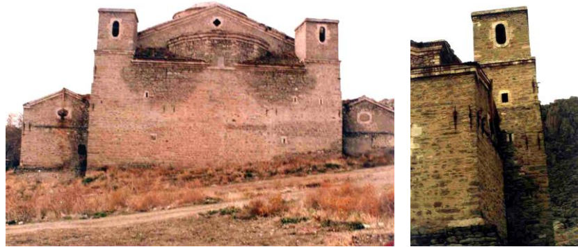
Figure 3.5 View of semi-demolished bell towers (ÇE-MİM, 2001)
