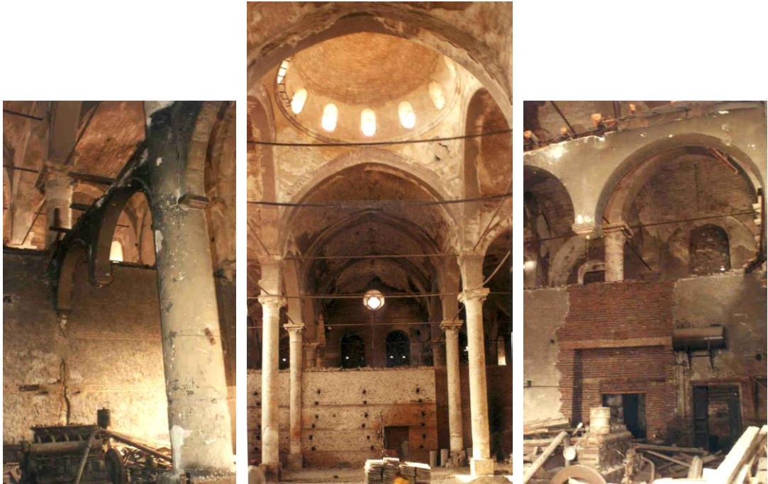
Figure 3.4 Additional walls included in the original state of the main hall, before the restoration works, (ÇE-MİM, 2001)
