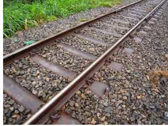
Source: Photographed by Study Team Figure 3-10 Ballast of Uneven Sizes
