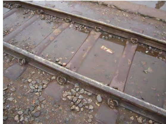
Source: Photographed by Study Team Figure 3-12 Track with Insufficient Ballast
