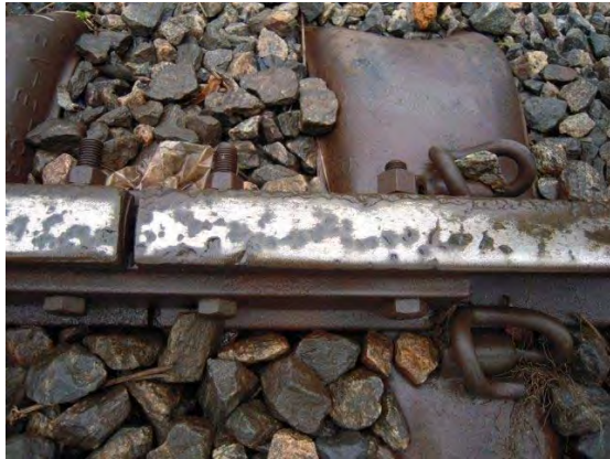
Source: Photographed by Study Team Figure 3-11 Damaged Rail
