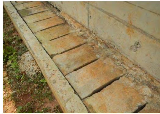
Source: Photographed by Study Team Figure 3-18 Concrete Duct
