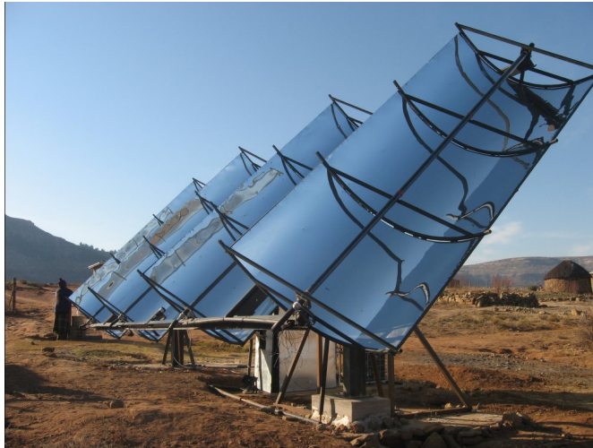
Figure 74: First solar ORC prototype, installed by STG in Lesotho, 2007
