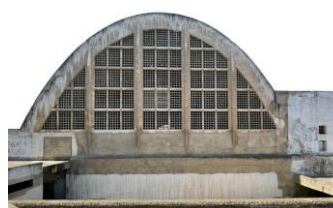
Figure 21. Decays on South Facade
