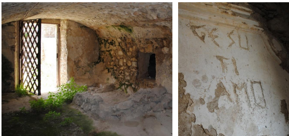
Figure 7. Examples of vandalism at the castle.
