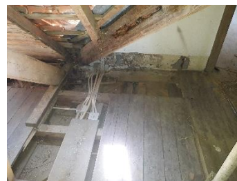
Figure 5. Leaks through the roof close to the turret (credits: Aníbal Costa)
