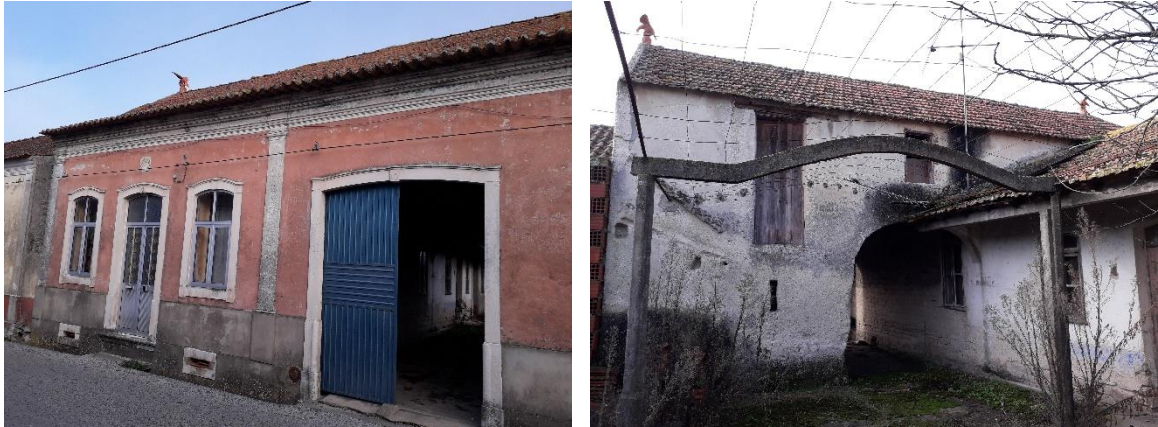
Figure 11. Front facade and interior view of the courtyard of Gandaresa House, Seixo, Mira (credits: Aníbal Costa)
