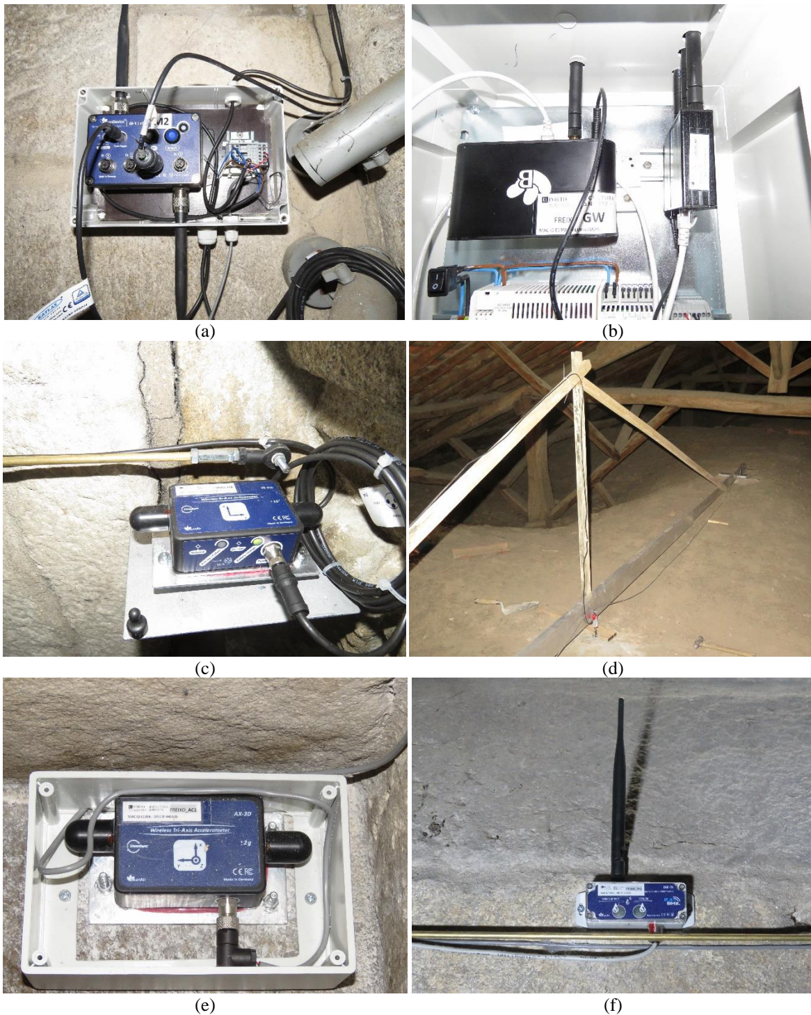
Figure 5. Monitoring system installed: (a) acquisition module M2; (b) gateway; (c) tiltmeter (CL2) and extremity of crackmeter FS3; (d) crackmeter FS7 installed on the extrados of the vault; (e) accelerometer (AC1); (f) temperature sensor TH1 and the extension rod of the crackmeter FS2 [source: authors].
