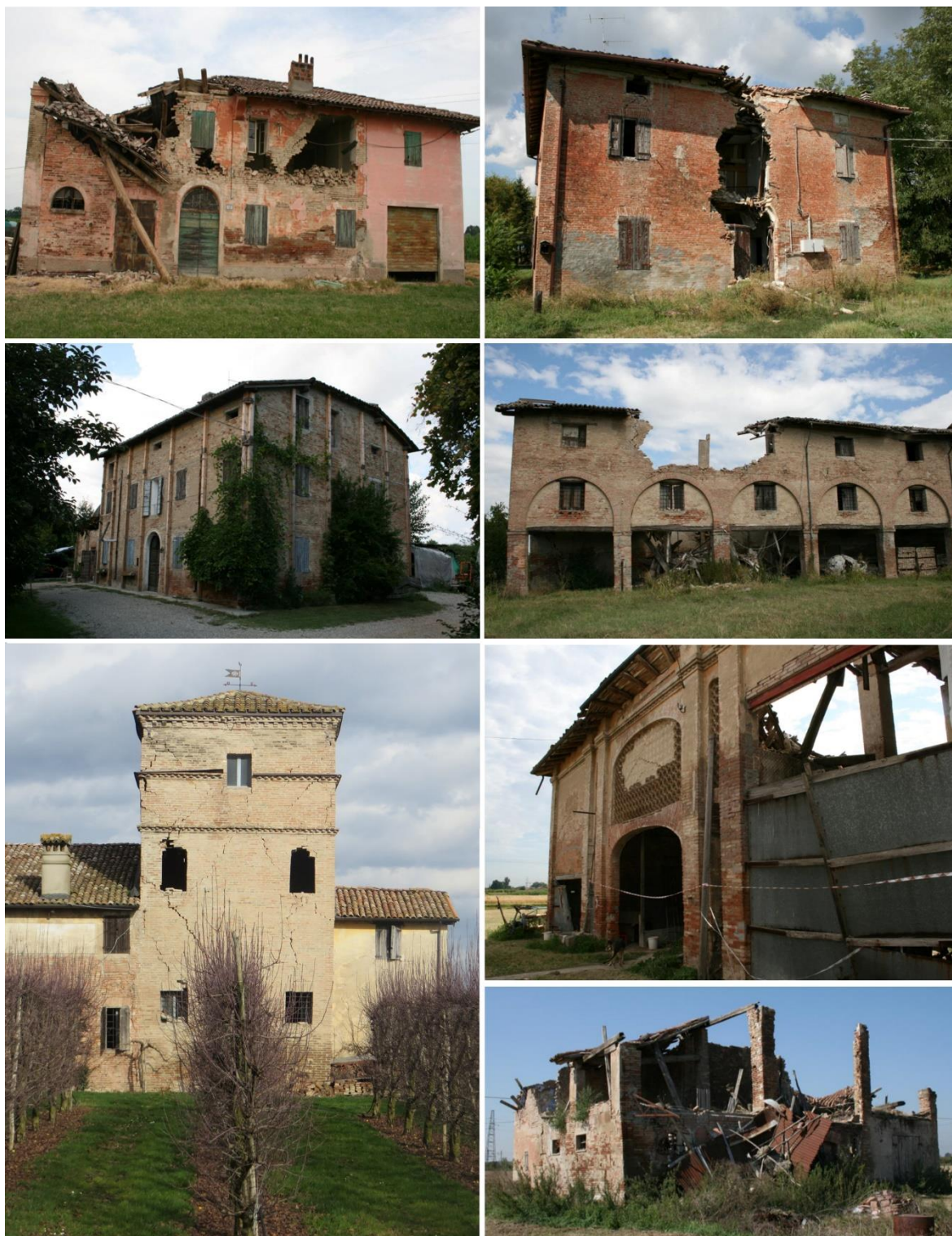
Figure 3. Spontaneous built heritage at the earthquake test: Crevalcore, Bologna ( top, centre, and bottom-right ); San Felice sul Panaro, Modena ( bottom-left )
