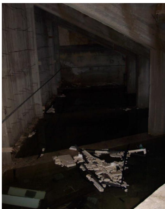
Figure 3. Foundation premises flooded
