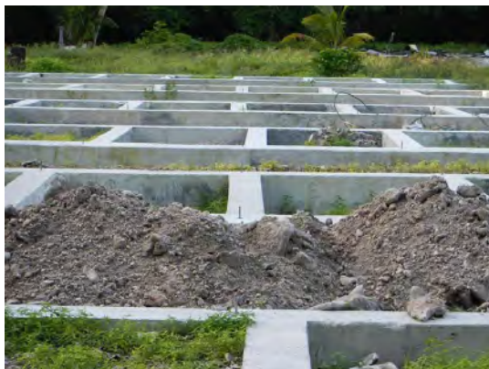
FIGURE 7: THREADED RODS CEMENTED INTO CONCRETE FOUNDATION. NOTE THAT THE RODS ARE LINED UP WHEREAS THE CONCRETE IS NOT.
