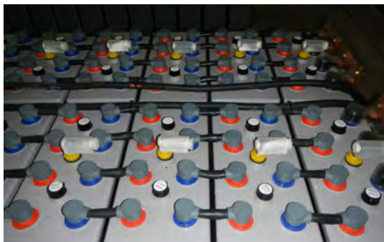
FIGURE 17: DETAIL OF THE TOPS OF THE BATTERIES. THE YELLOW AND WHITE CAPS ARE THE CATALYTIC COMBINER CAPS, AND THE BLACK CAPS ALLOW OPERATORS TO ACCESS THE BATTERIES TO TOP THEM UP WITH DEIONIZED WATER.
