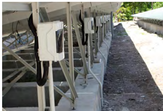
FIGURE 10: ALL ARRAY ISOLATOR ENCLOSURES ARE LOCATED UNDER THE PANELS TO SHIELD THEM FROM THE SUN AND RAIN.
