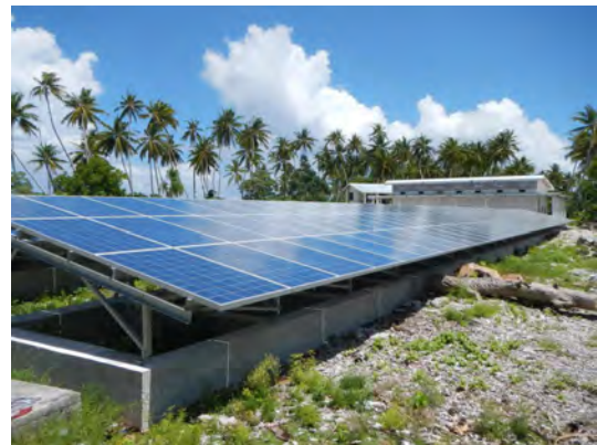
FIGURE 9: FRONT ROW OF PANELS ON NUKUNONU. THE PINK BUILDING IN THE BACKGROUND IS THE PURPOSE-BUILT BATTERY BUILDING.
