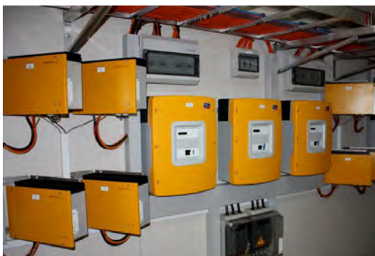
FIGURE 13: THE 3 BATTERY INVERTERS AND THE 4 CHARGE CONTROLLERS IN A CLUSTER. THE CONFIGURATION FOR THE FAKAOFO INVERTER ROOM WAS DIFFERENT FROM THAT FOR THE NUKUNONU AND ATAFU INVERTER ROOMS (DUE TO DIFFERENT BUILDING LAYOUTS)
