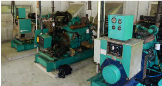
FIGURE 18: THE THREE GENERATORS ON FAKAOFO. AT THE TIME OF INSTALLATION OF THE PV SYSTEM, ONLY TWO OF THESE WERE OPERATIONAL. NUKUNONU AND ATAFU ONLY HAD ONE OPERATIONAL GENERATOR EACH.
