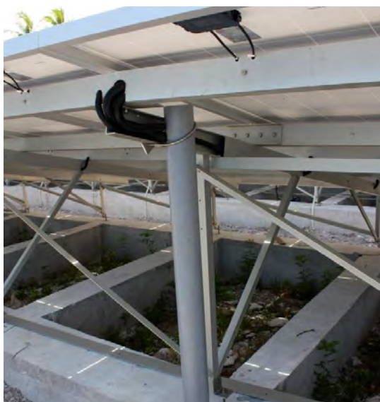
FIGURE 11: ALL CABLES ARE PROTECTED IN UV-RESISTANT CONDUIT OR ALUMINIUM CAPPING
