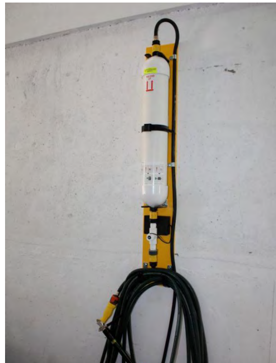
FIGURE 16: THE DEIONIZER IS USED TO PROVIDE WATER FOR TOPPING UP THE BATTERIES' ELECTROLYTE LEVELS.
