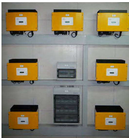
FIGURE 12: THE STRING INVERTERS IN A CLUSTER, WITH THE AC AND DC ISOLATORS IN THE MIDDLE.
