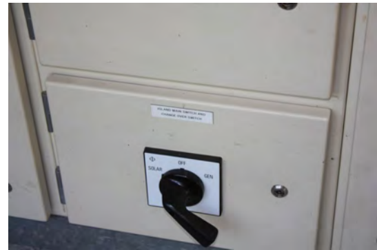
FIGURE 20: THE CHANGEOVER SWITCH ON ATAFU
