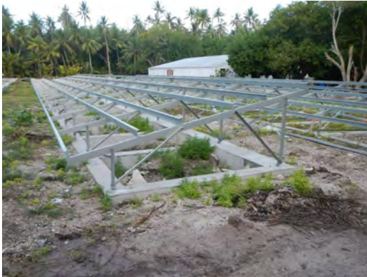
FIGURE 8: ALUMINIUM MOUNTING STRUCTURE ON FAKAOFO. THE BUILDING IN THE BACKGROUND HOUSES THE BATTERIES AND THE INVERTERS.
