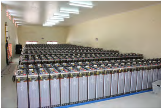
FIGURE 15: THE BATTERY ROOM ON ATAFU. EACH BANK OF BATTERIES HAS A NAMEPLATE STORAGE CAPACITY OF 288 KWH.
