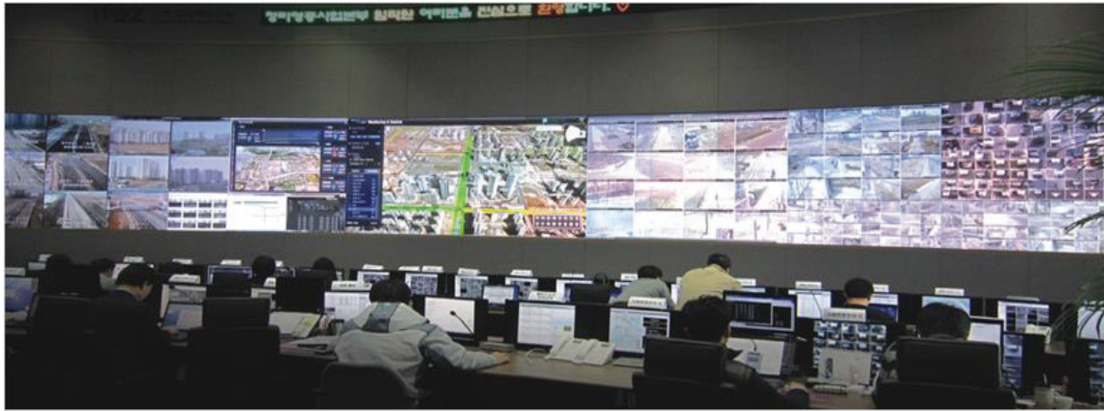
Figure 18 View of IFEZ(Songdo U-city) Integrated operation center
