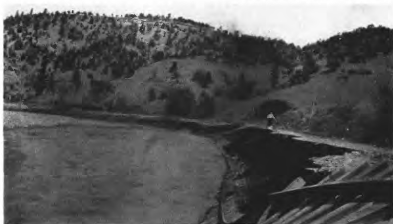
DAMAGE TO TRACKS OF DENVER & RIO GRANDE RAILROAD CAUSED BY FLOOD OF OCTOBER 1911 ON SAN JUAN RIVER NEAR PAGOSA JUNCTION.
