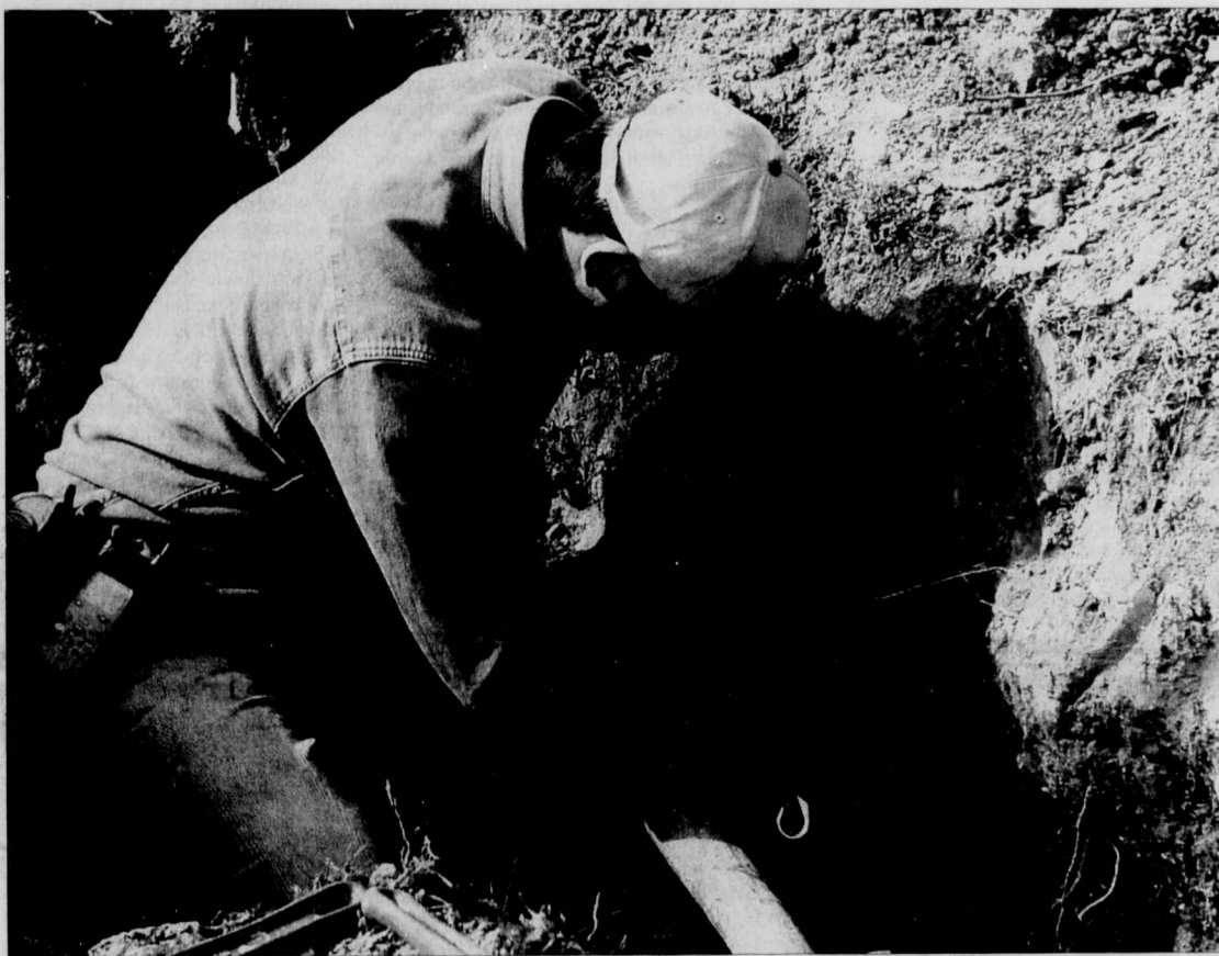
A maintenance worker at the Park Ridge Apartments works to find a natural gas leak that has caused hundreds of residents to go without hot water for more than a week.
