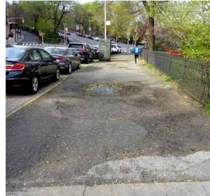
Before: The pavement in this area was weathered and deteriorating.
