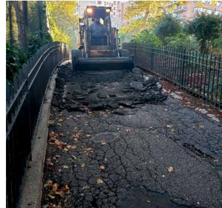
Breaking up and removing the old pavement on the pathway to Jenny's Garden at 139th Street.
