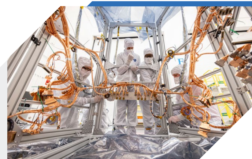
With almost 2,100 feet of wiring, the electrical harness on Europa Clipper’s propulsion module is one of the largest APL has ever built.
