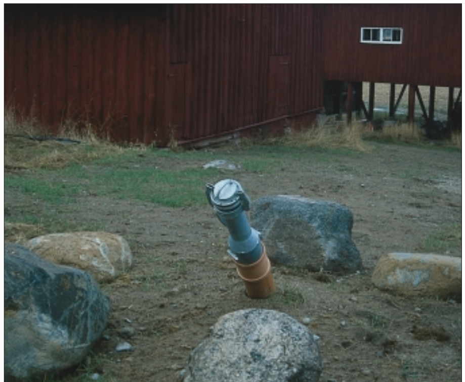
Connection pipe used by tank trucks to fill the storage tanks at Lake Bornsjön.
