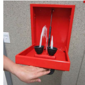
Figure 5 Eyewash station inspection
