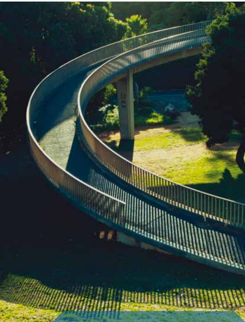
A pedestrian bridge (part of the railing stolen for scrap) near Cape Town, South Africa
