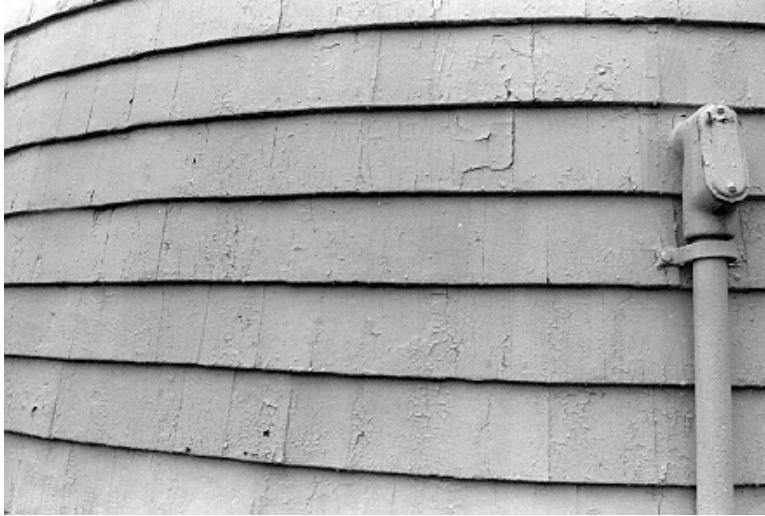
Figure 15. View of Class III paint condition: in this case the cracking, peeling, and alligatoring have been caused by excessive paint layer build up.
