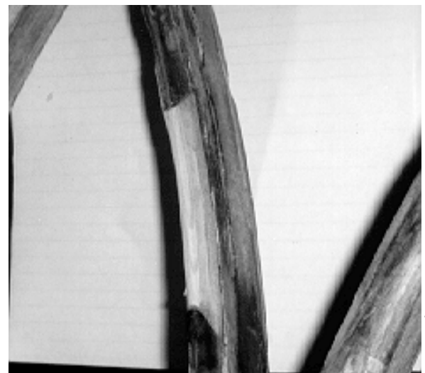
Figure 13. Close-up of a dutchman repair (light-colored wood used to mend a window muntin).
