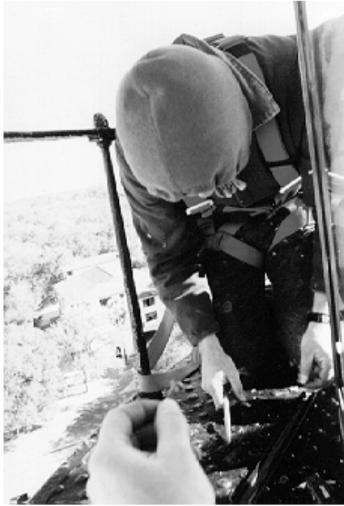
Figure 17. Note the detailing of the finished exterior astragal in place and the polybutyl sealant tape visible in profile.
