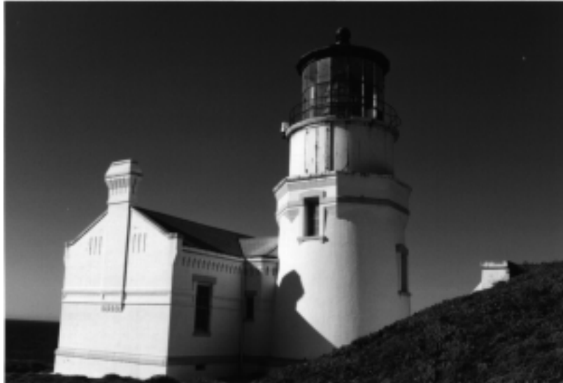
Figure 44. Before the rehabilitation. Note the doors at the watch room. A new louvered panel will be installed for added ventilation.
