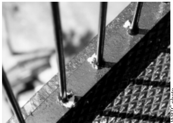
Figure 40. The paint on this stainless steel replacement gallery deck has begun to peel less than three months after it was painted. This could have been prevented if the stainless steel parts were first cleaned and then lightly glass-bead blasted.
