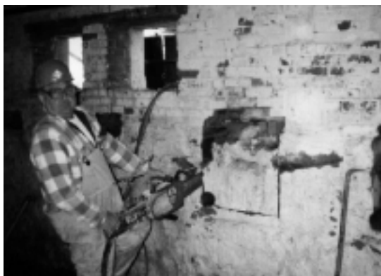
Figure 15. A hydraulic chain saw with industrial diamond teeth is being used to cut openings below the grade line for insertion of the steel beams.
