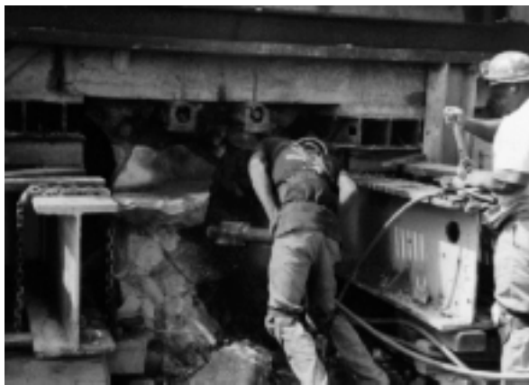
Figure 19. Once the initial lift was performed, the remaining foundation between the beams was removed.
