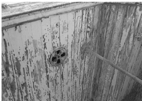
Figure 13. The paint coating that once protected this lantern parapet wall has failed.
