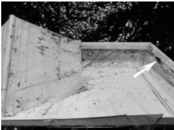
Figure 9. View of built-in gutter system on a mansard-style roof; the arrow indicates where a fist-size hole exists. This hole allows water to enter the interior of the lighthouse.
