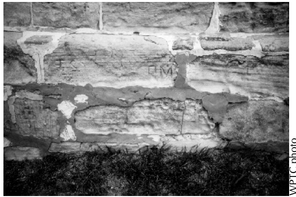
Figure 19. The use of hard portland cement mortar and sloppy pointing technique have aided in the deterioration of this soft sandstone wall.
