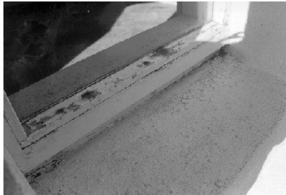
Figure 9. Rust occurring on the inside of the steel channel that forms the sill of this metal casement window.
