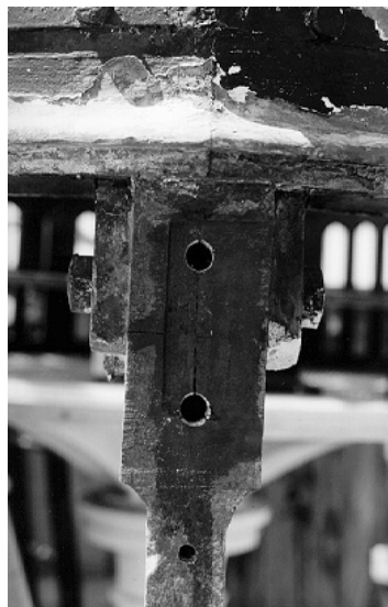
Figure 36. View of the gallery bracket tenons after the holes have been drilled. The tenon on the right connected to the exterior gallery; the tenon on the left is part of the interior gallery deck bracket. The 'v' that has been stamped in the end of the left tenon is an assembly identification mark.
