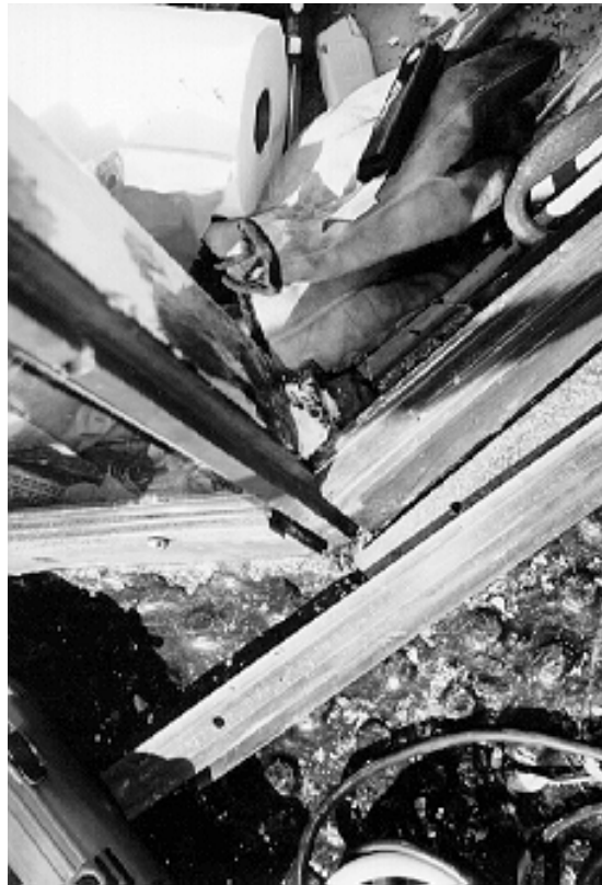
Figure 14. Following placement of the restored bronze mullion, the fenestration is ready to receive the new glazing system.
