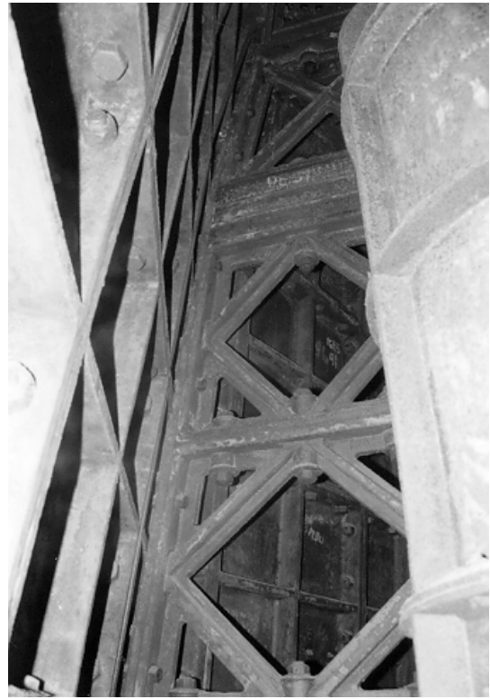
Figure 6. A view of the inner cavity and skeletal structure of the Cape Henry Lighthouse.
