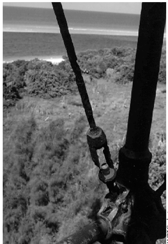
Figure 16. As corrosion attacked this steel turnbuckle, wind and airborne sand eroded away the flaking rust.
