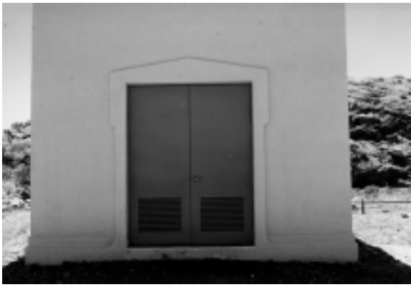
Figure 11. These replacement lighthouse doors have screened louvers that cover approximately 25% of the door opening to maximize air exchange.
