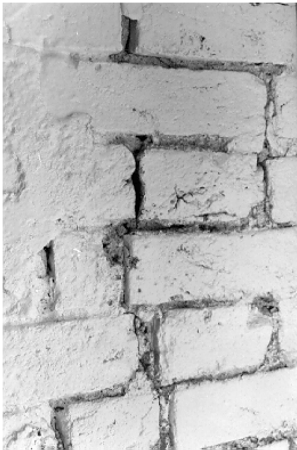
Figure 21. Detail of eroded pointing.
