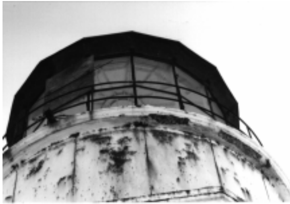
Figure 46. Lighthouse lantern before rehabilitation. Note the missing ladder rails and the severe rust on the lantern cornice and lower watch room panels. The badly spalled concrete gallery deck was installed in 1947 and is not original.
