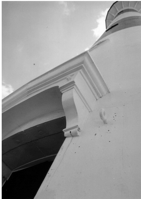
Figure 45. Within three months after painting, the rust began to bleed through this weep hole on the bottom of this pediment bracket. Two lessons are to be learned from this condition: 1) keep weep holes open to allow any water that may have entered the casting to escape, and 2) keep joints around applied castings sealed; apparently this was not done and water has entered the hollow cavity of the pediment, causing rust to form inside.
