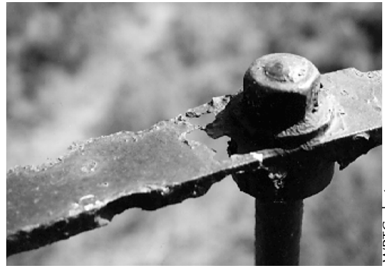
Figure 15. As corrosion attacked this steel handrail, wind and airborne sand eroded the loose and flaking surface rust.
