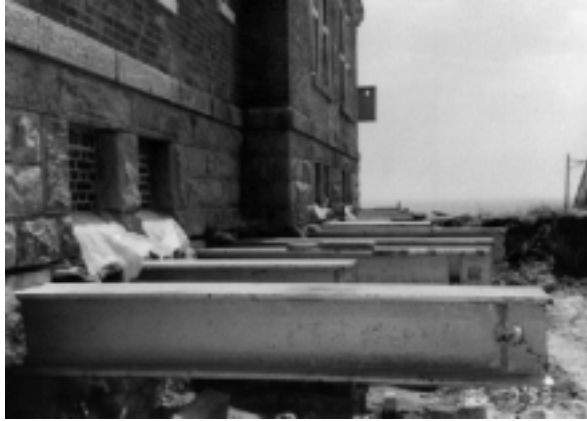
Figure 18. Large cross steel beams are inserted into the cut opening to form part of the grid that will carry the building.
