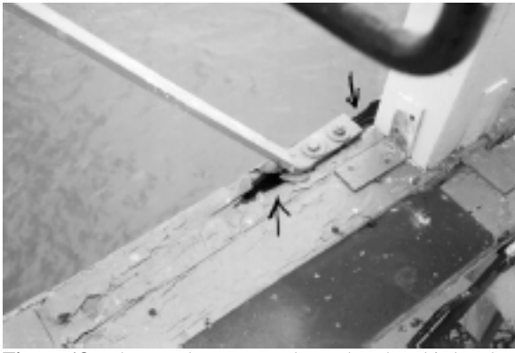
Figure 18. The wooden structural member that this bracket is attached to is extensively deteriorated. This condition is a prime example of deterioration that can be repaired by cutting back the rotted wood to a sound substrate, then fitting the void created with a wooden ‘dutchman’ or infill that matches as closely as possible the grain orientation and wood species as the existing member. Once the dutchman has been glued, and if needed, doweled in place, then the affected area should be properly primed and painted. This technique is affordable and incurs only minimal damage to the existing historic materials.
