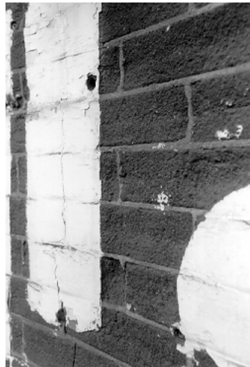
Figure 17. Deeply eroded brick as a result of sandblasting. The white areas are where electrical components were attached to the wall at the time of sandblasting.
