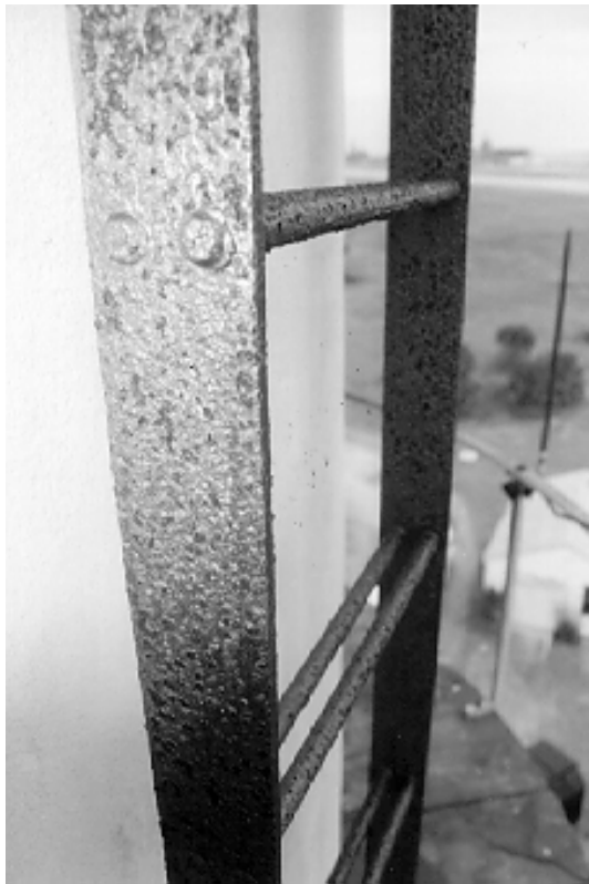
Figure 11. Detail view of a steel ladder that has been uniformly attacked by corrosion.
