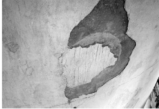
Figure 26. Once the scaffolding was erected, areas of the delaminated white mortar finish coat were removed.
