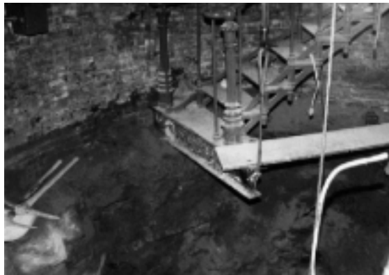
Figure 14. The concrete floor of the light tower was removed and earth excavated by hand in order to perform stabilization from the interior of the structure.
