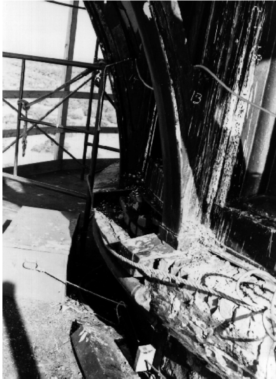
Figure 16. At the base of the brackets, the cast-iron belt course is removed, exposing deteriorated masonry below.
