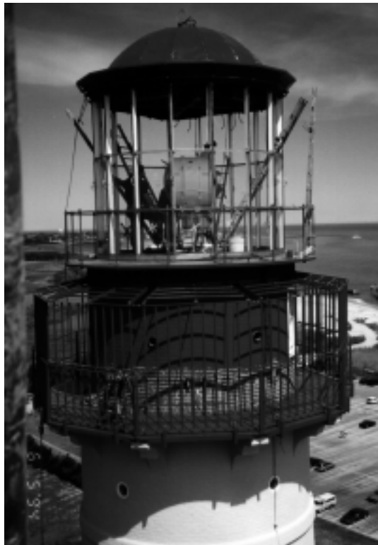
Figure 9. The refurbished roof is replaced on the lantern room. The fit is almost exact.
