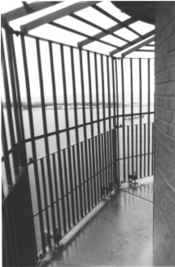
Figure 25. To protect visitors from falling or jumping from a lighthouse tower, a safety railing system or ‘cage’ is often built around the gallery decks. The cage at Barnegat Lighthouse was designed so that it has minimal impact on the historic structure and can be removed with little, if any, damage to the original fabric. Note that the cage is also enclosed to prevent climbing over the top.
