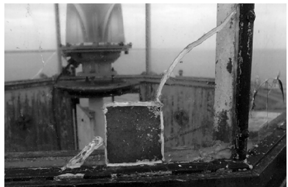
Figure 6. An acceptable temporary lantern glass repair made using a small piece of sheet metal and caulking.
