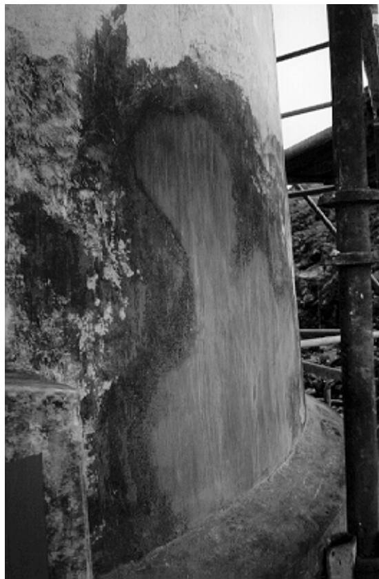
Figure 27. The areas where the loose mortar finish coat was removed were repaired with a two-part mortar patch. The final texture on the patch was tooled to match the historic wall surface. The patch was completely invisible after the tower was painted.
