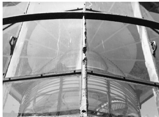
Figure 14. Wind and airborne sand have accelerated the deterioration of this lantern gallery deck handrail
