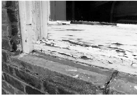
Figure 8. Deterioration of the bottom rail and sill on a wooden double-hung window.
