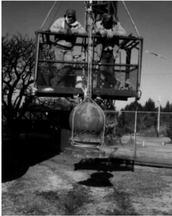
Figure 4. The first step in removing the roof was to take off the vent ball. The vent ball not only serves as a lightning rod but also provides ventilation to the glass in the lantern room, limiting condensation.
