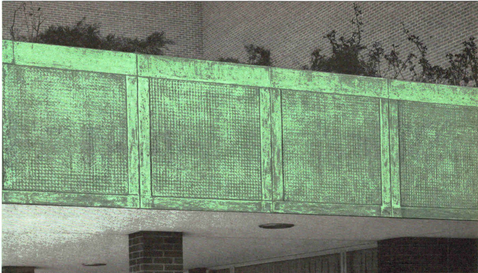
McMorran Memorial Auditorium, Port Huron, Mich. Architect: ALDEN DOW, Midland, Mich. General Contractor: COLLINS & CATLIN, INC., Port Huron. Fabricators and Erectors: MAUL MACOTTA CORPORATION, Detroit.
