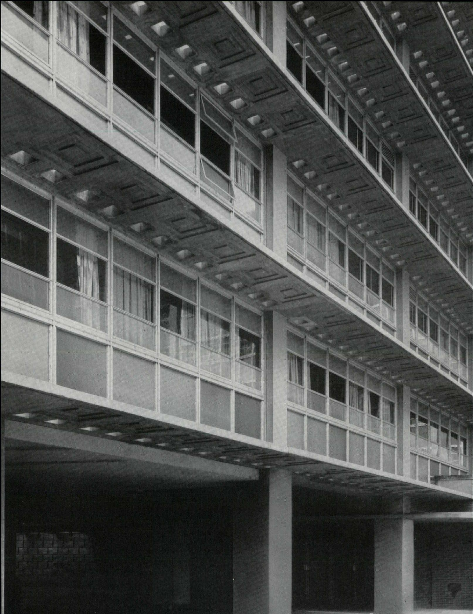
DECORATIVE MULLION PATTERNS and sharp, clean exposed holes are formed in cantilevered floor slabs at the University of Arkansas Medical Center, Little Rock. The job was performed easily and economically with little finishing required — one of the many "plus" advantages
