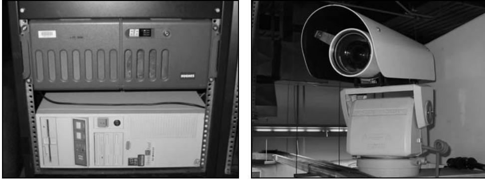
Figure 4. Autoscope Supervisor PC (bottom on left) and the Autoscope camera as installed.
