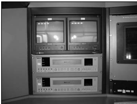
Figure 5. Video surveillance system as installed in the operator console.
