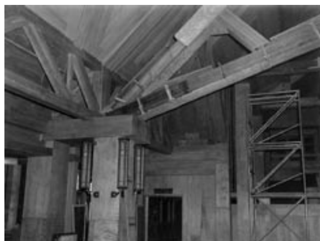
The structural failure in the roof trusses of the Canyon Hotel lobby was caused by foundation problems.
