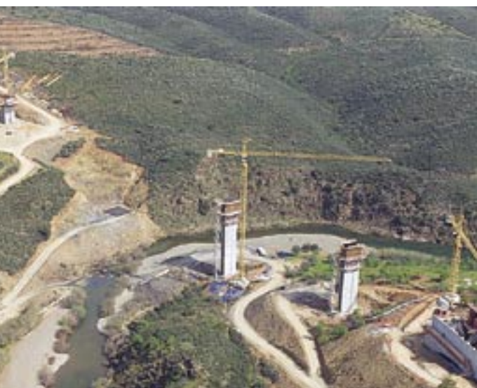
IEP – IC27 – Odeleite / Alcouthim (Viaduto da Foupana) – Motorway IC27 – Odeleite / Alcouthim (Foupana Viaduct)
