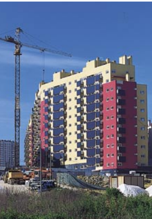
JARDINS EXPO – Construção dos Lotes RTB6 e RQ3 nas Olaias, Lisboa – Construction of Housing Buildings, Lots RTB6 and RQ3, at Olaias, in Lisbon
