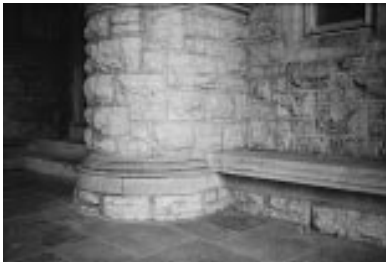
Column base transitions into a thoughtful detail which weathers well and allows a graceful visual transition from the vertical column to the ground plane.
