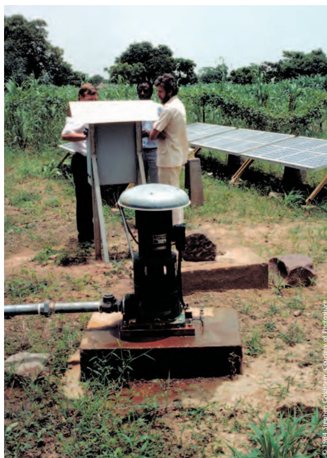
Solar water pumping in Mali
