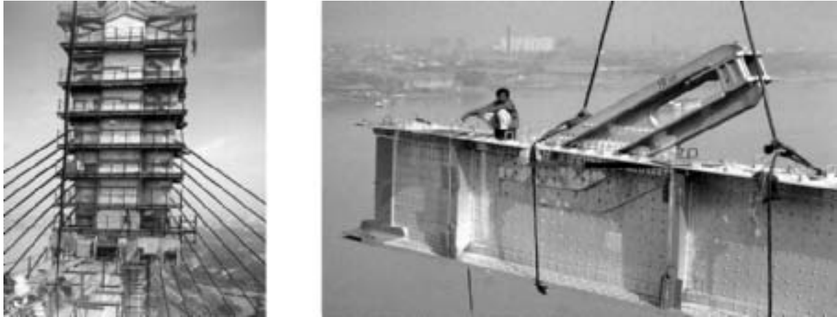
Fig. 4.33: Calcutta bridge, Schlaich. “Flower pot” type pylon anchorage design. Normally tendons are prestressed at deck level. It was decided to prestress the tendons on the pylon to ensure quality control and to facilitate inspection. The steel was riveted together by local labor. (Holgate)
