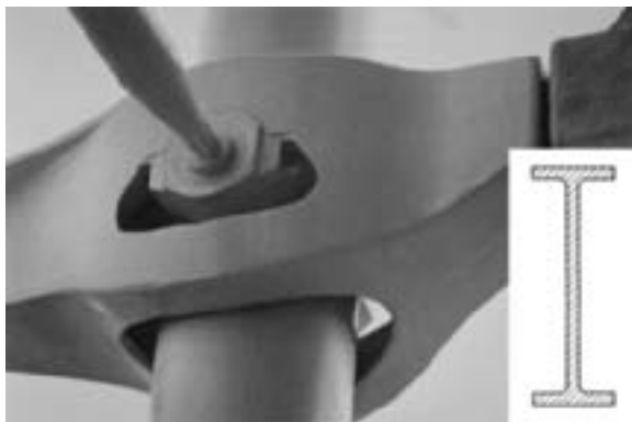
Fig. 4.23: Cast steel giberette at connection, Pompidou Centre, Paris, compared to a standard, rolled I-beam. (Dunster; Mainstone)
