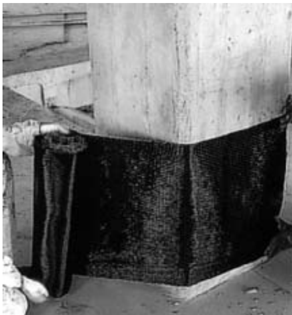
Fig. 6.18: Example of FRP sheet reinforcement of existing reinforced concrete bridge pier. (CCLab, after Sika)
