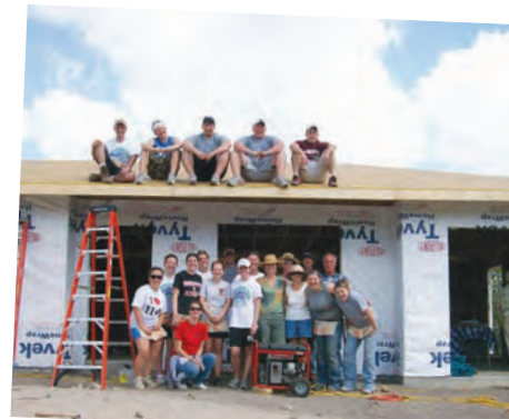
Members of G.I.V.E. spent their spring break in Port Charlotte, Florida with Habitat for Humanity last March building the shell of a home from the ground up.
