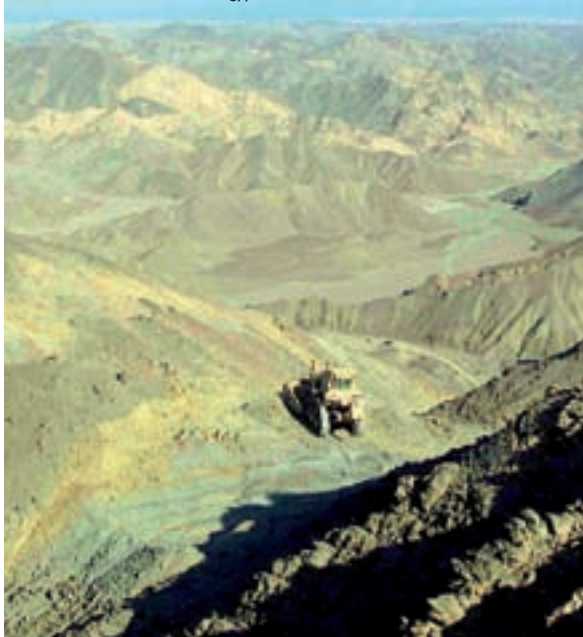
Gippsland Minerals at work: Preparing the laydown area on the 440RL at the Abu Dabbab mine in Egypt
