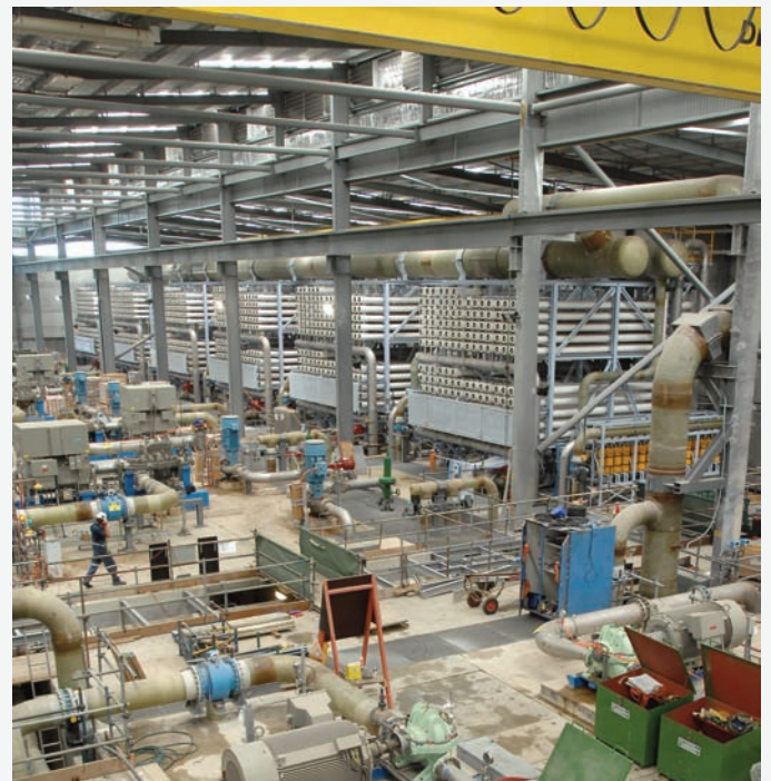
Inside view of the Perth SWRO Desalination Plant.
