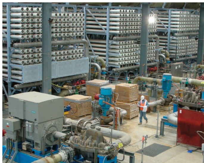
Membrane racks tower over the small footprint of the PX array train racks.
