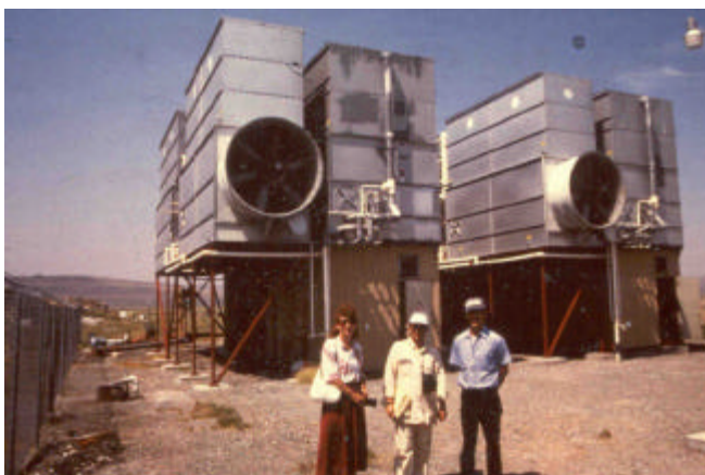
Figure 21. Wineagle binary plant of 2x375 kW in northern California, USA.
