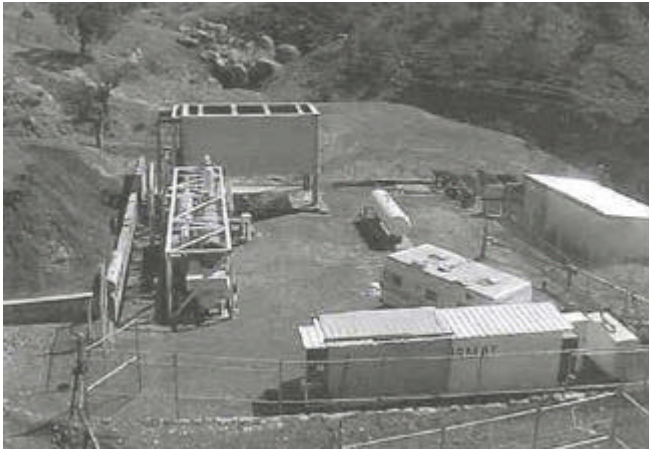
Figure 20. 300-kW binary plant at Maguarichic, Mexico (courtesy of CFE).
