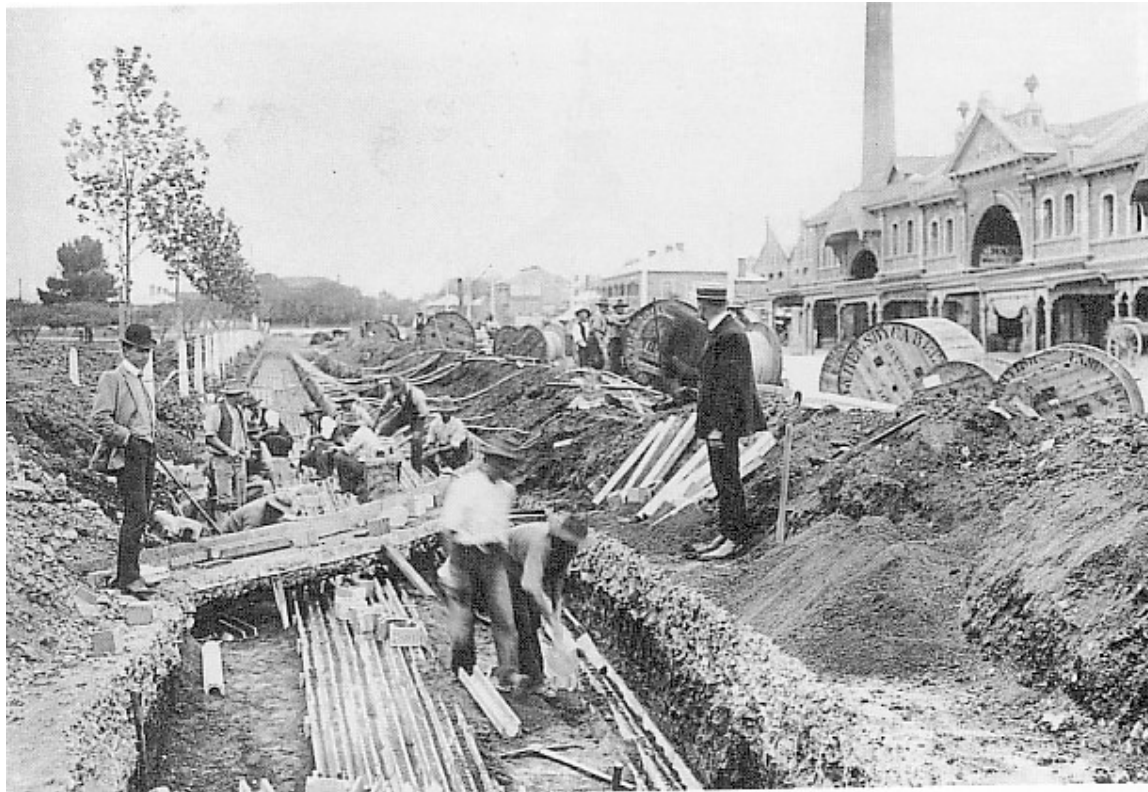
Image: Laying electricity cables in East Terrace in 1907-08. Note the white painted post and wire fencing and the young Plane Trees ( Platanus orientalis ) to the left. Source: NSW State Library.
